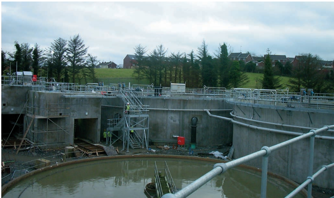
Construction of CASS™ basins & inlet works at western end of site (courtesy: Earth Tech Engineering Ltd)
