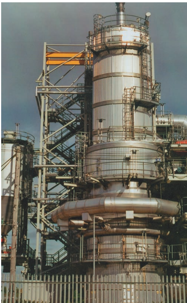
Knostrop Incineration plant showing incinerator stack with Ash hopper to left (courtesy Arup)
