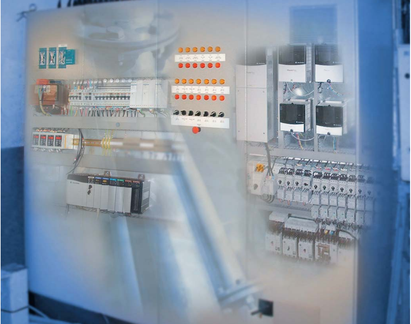
Nanstallon Sludge Processing Centre is controlled by an integrated control system using Rockwell Automation components.
