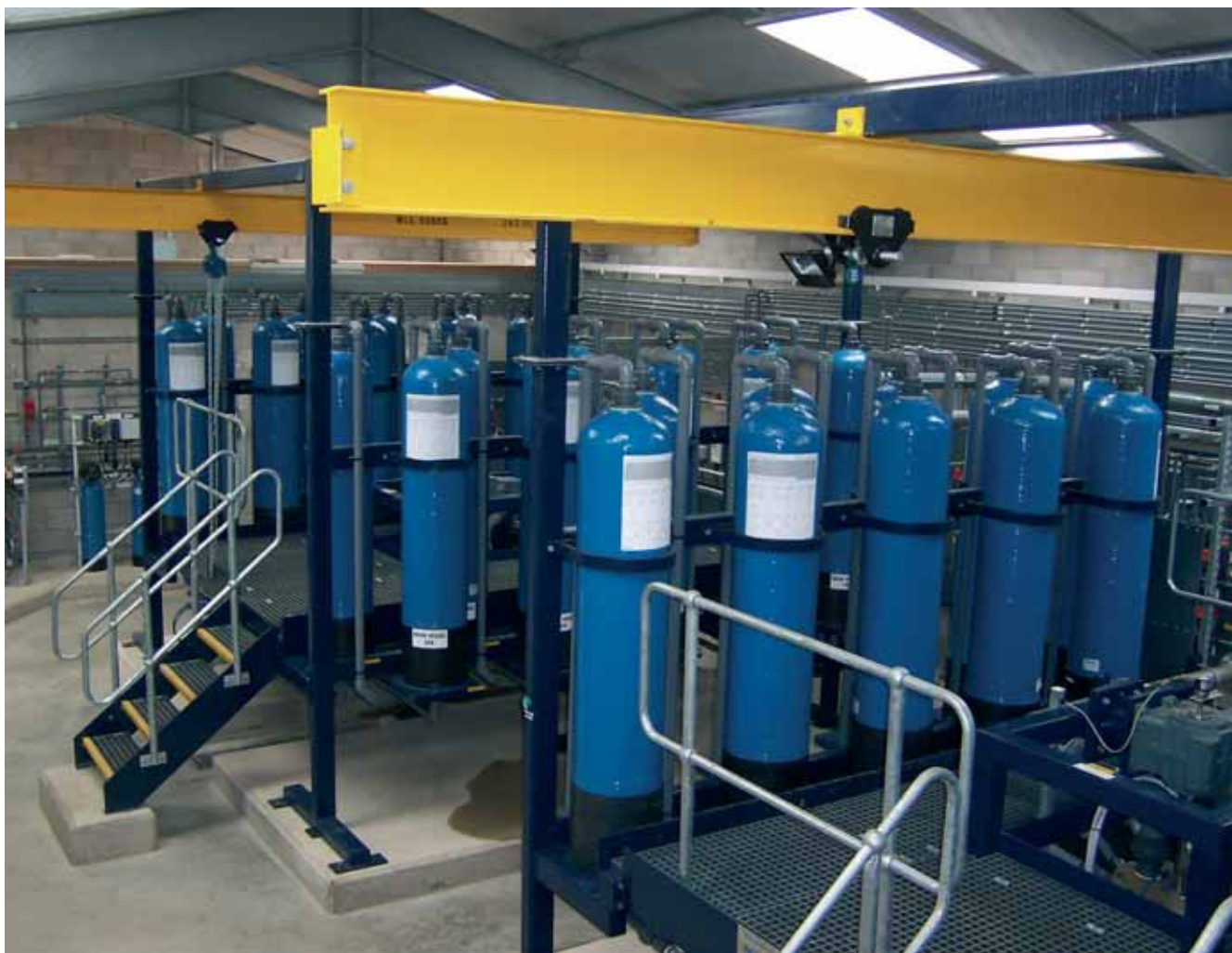
NITREAT system installed at Sheafhouse WTW for Thames Water
