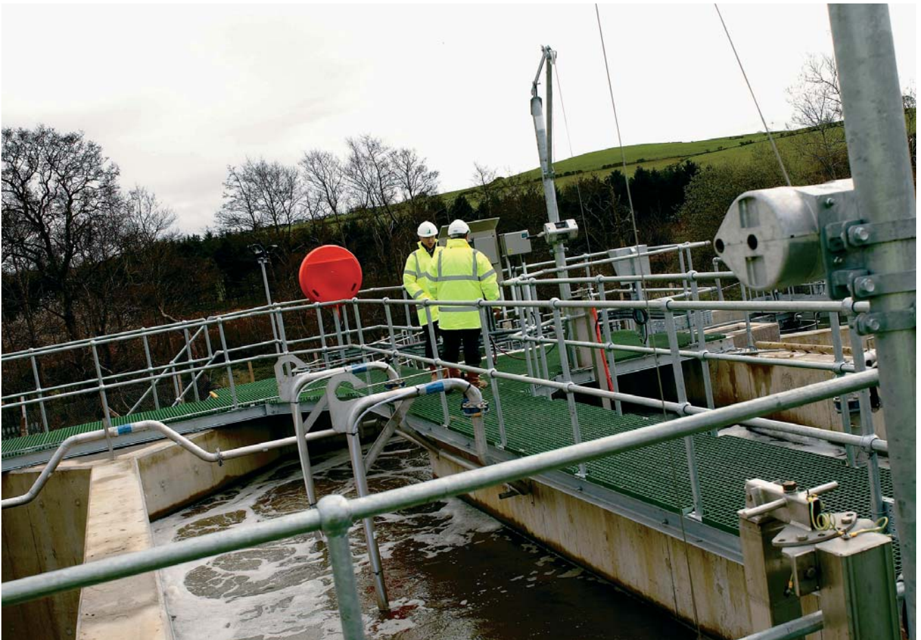
IBA Lanes at Claudy WWTW
