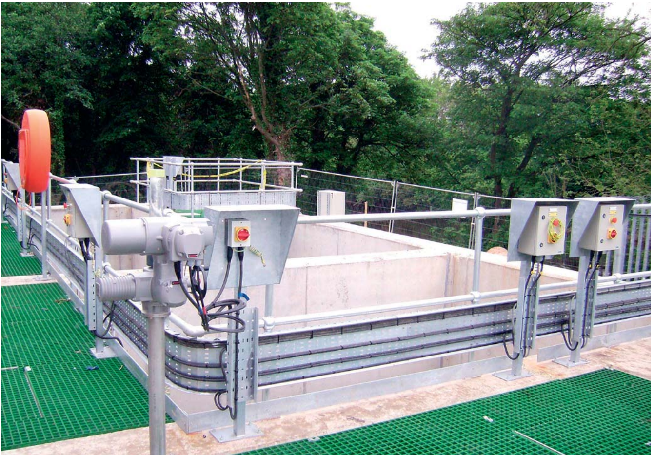
Storm Tank at Sion Mills WWTW
