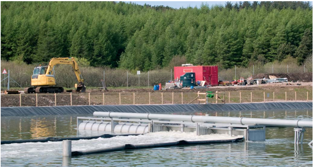
Tobermory: Diffuser provides aeration in the facultative primary lagoon
