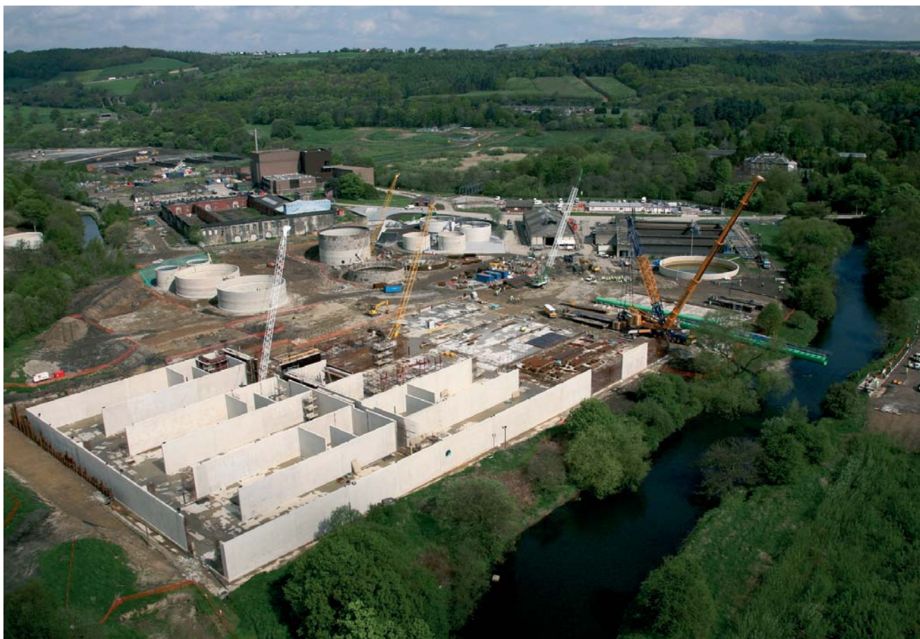
Esholt activated sludge tanks under construction. The large crane is installing a pipe bridge across the river connecting the ASP to the new final settlement tanks.
