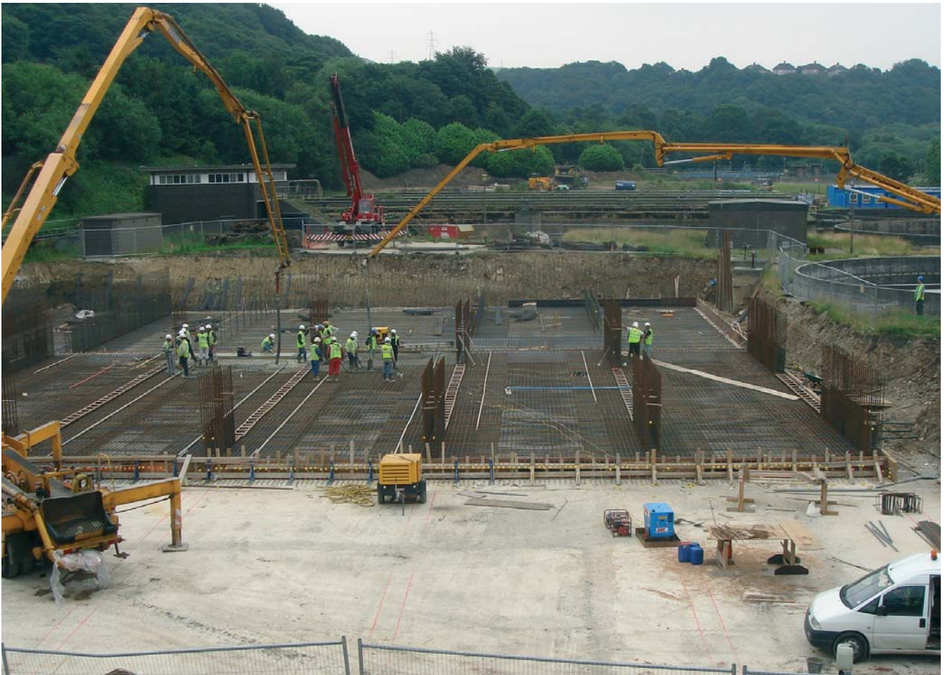
Halifax WwTW at 5am, July 2006 awaiting first delivery of concrete for the second pour for the new activated sludge plant
