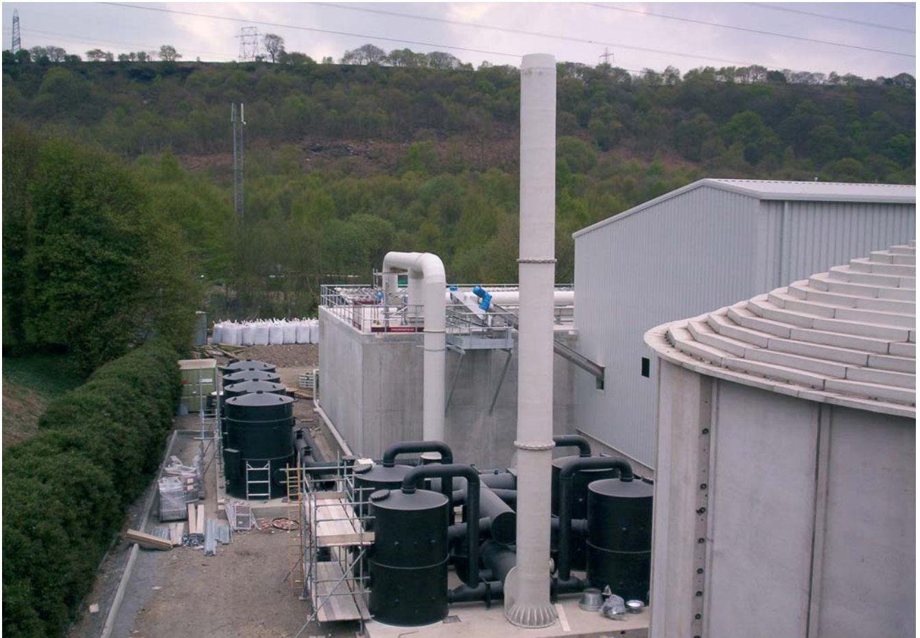
New odour control equipment installed at Halifax WwTW comprising bio-filters and carbon filters for sludge dewatering and storage facility.
