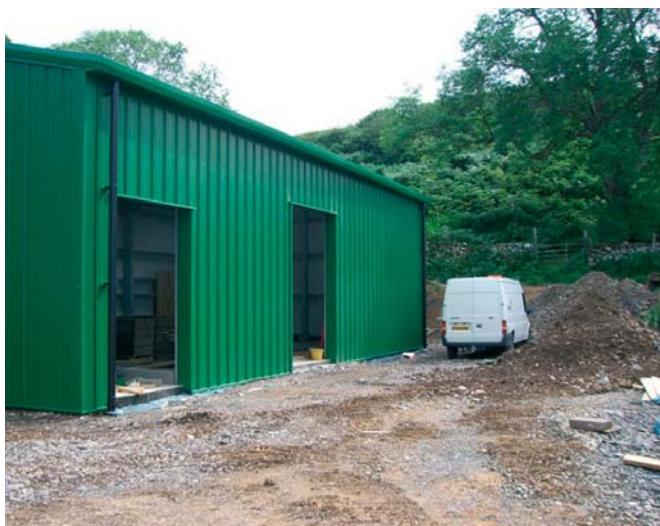
Water treatment building at Kilmelford
