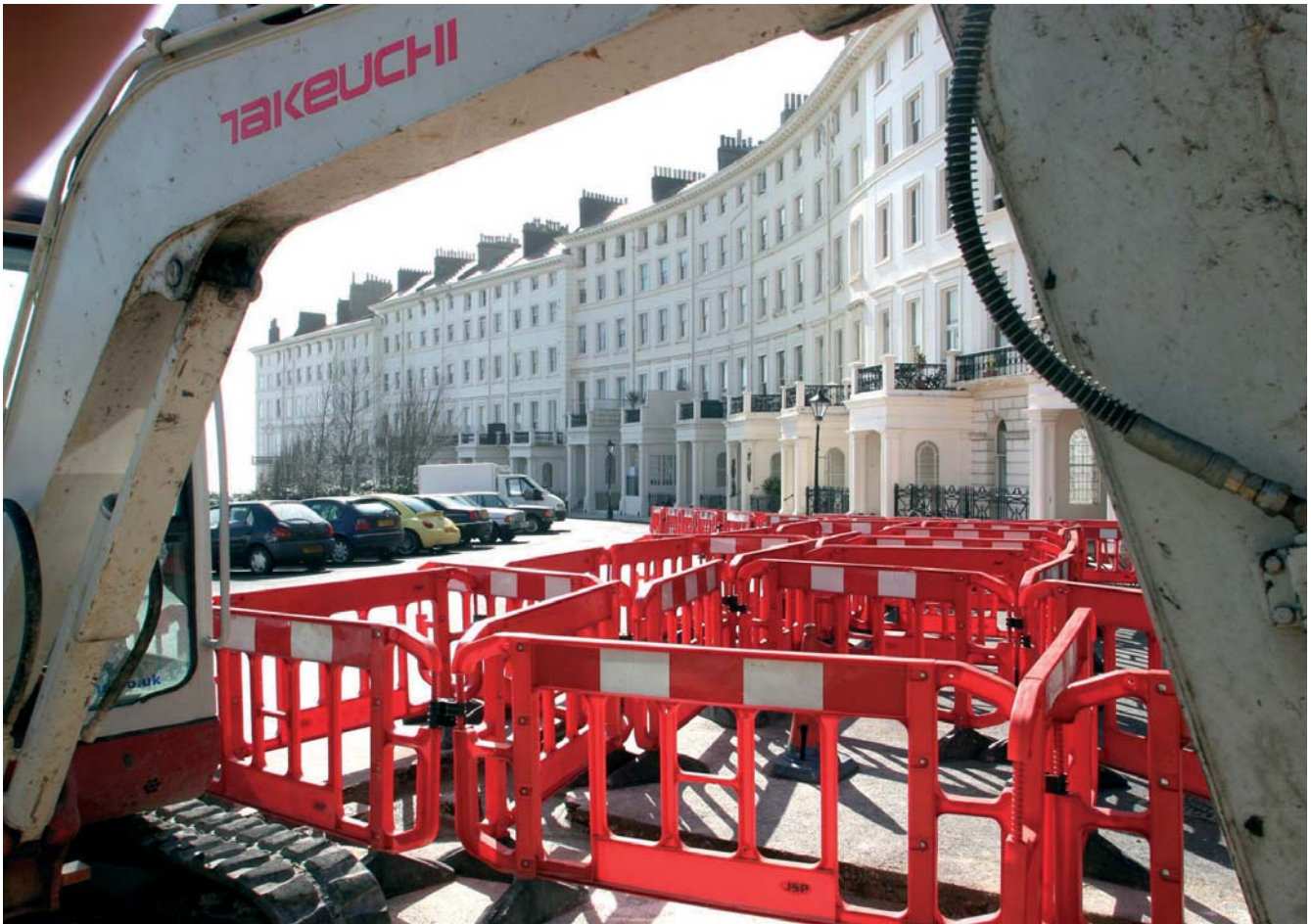
Digging techniques took into consideration the conservation of Regency Buildings in Brighton
