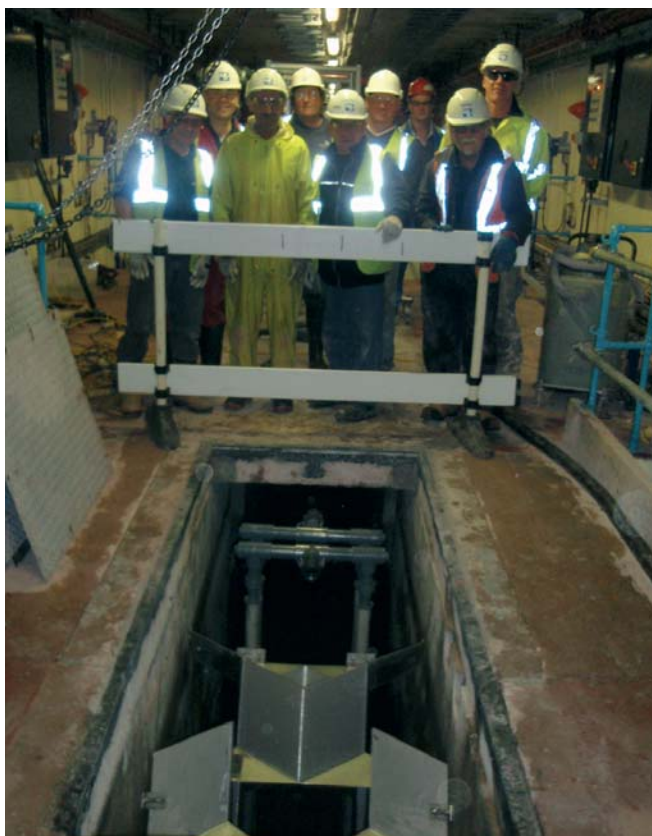
Completed installation of Chlorine static mixer Courtesy of Black & Veatch after only 2 No 6 hour shut downs of flows
