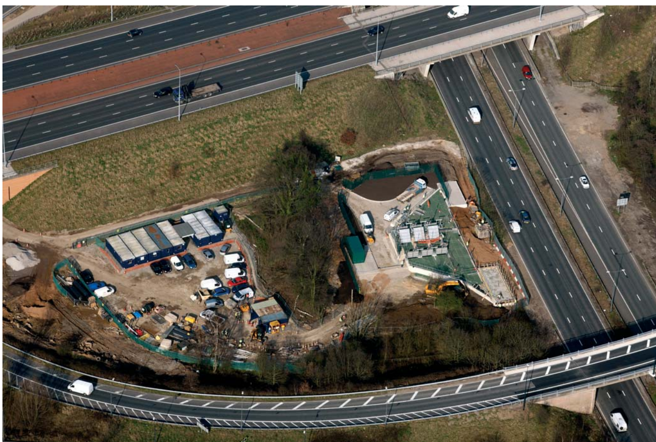
Princess Parkway Screening Chamber
