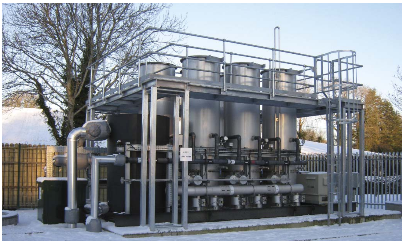
Tertiary sand filter treatment
