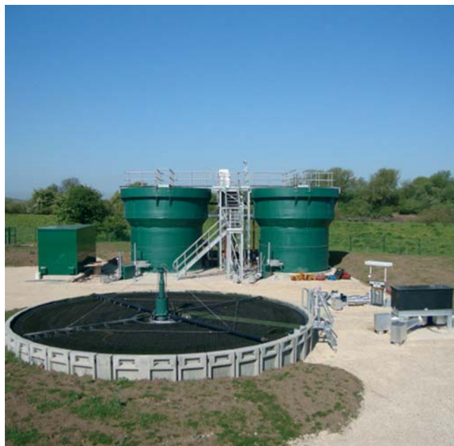
Glass reinforced plastic humus tanks in the background, with plastic media-percolating filter in the foreground Courtesy of CostainMouchel
