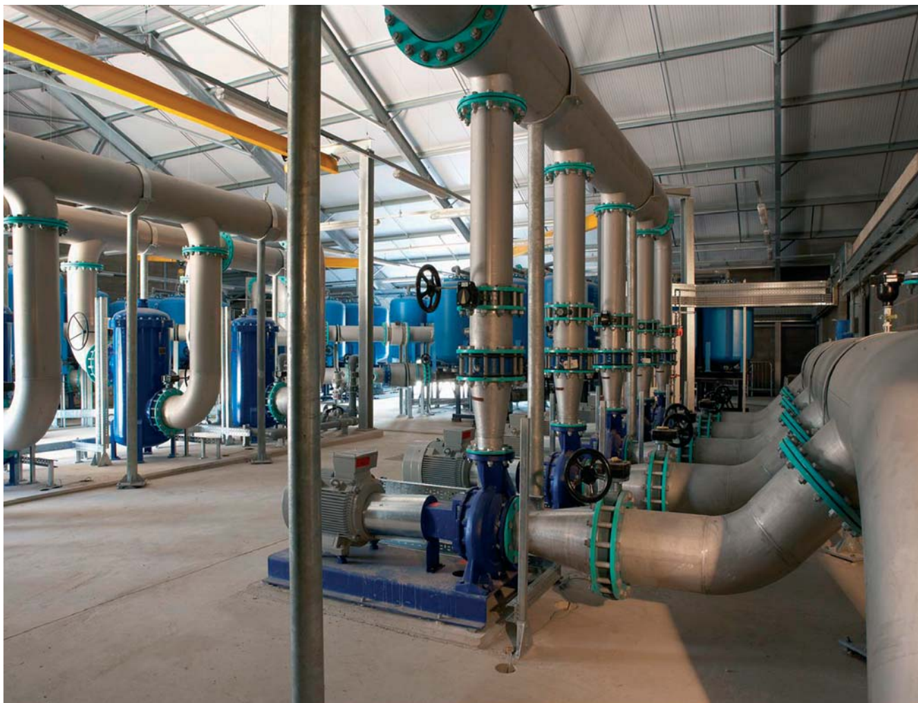
Feed Pumps & Bollfilters with Ion Ex Resin Vessels in Background
