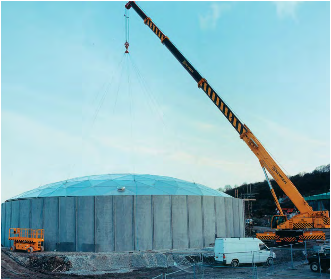
Falmouth CSO improvements - Raising the roof on the 6000m 3 storage tank (photo: Still Imaging, Chudleigh, Devon; courtesy S.W. Water)
