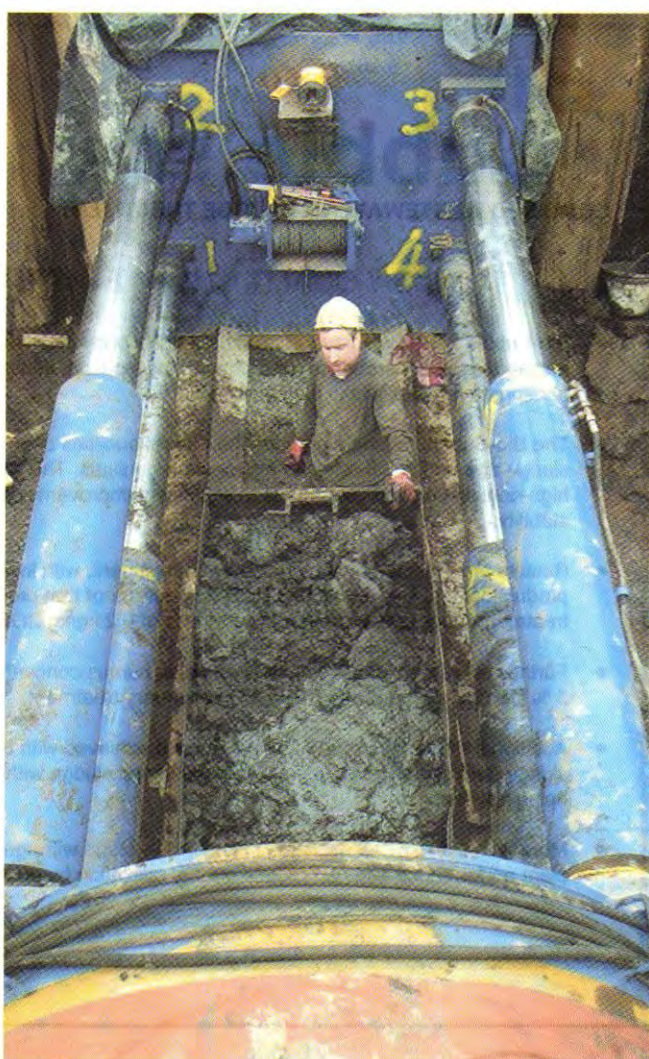
Hornsea Pumping Station (Courtesy Earth Tech Engineering Ltd)
