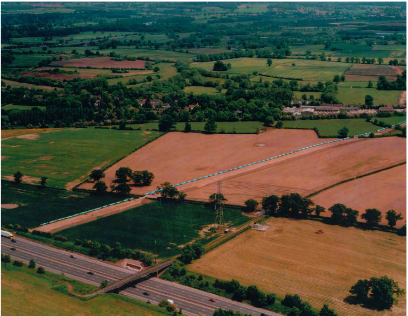
1200mm Ductile iron pipes ready to be laid (courtesy Severn Trent Water)
