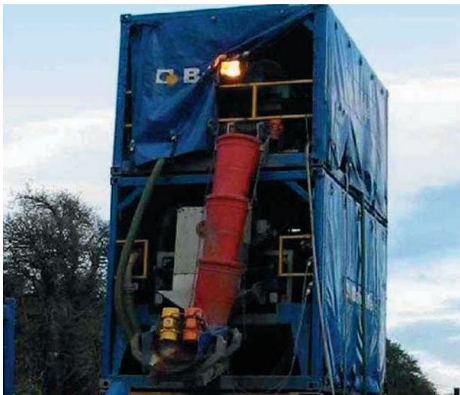
Separation plant in use at Bewdley (courtesy Barhale Construction).
