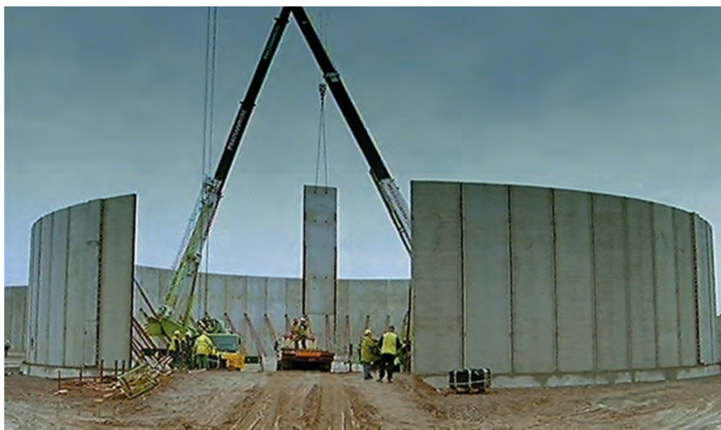
Final wall installation 12/12/02 (Time lapse photography by John Adderley, courtesy MJ Gleeson).
