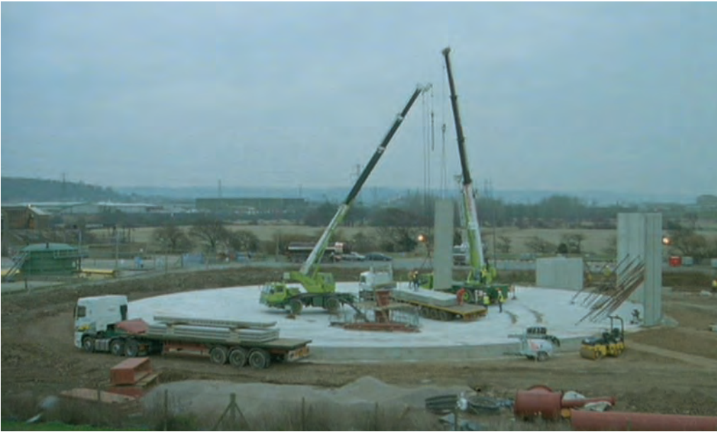
Photo shows start of construction 9/12/02 (Time lapse photography by John Adderley, courtesy MJ Gleeson).
