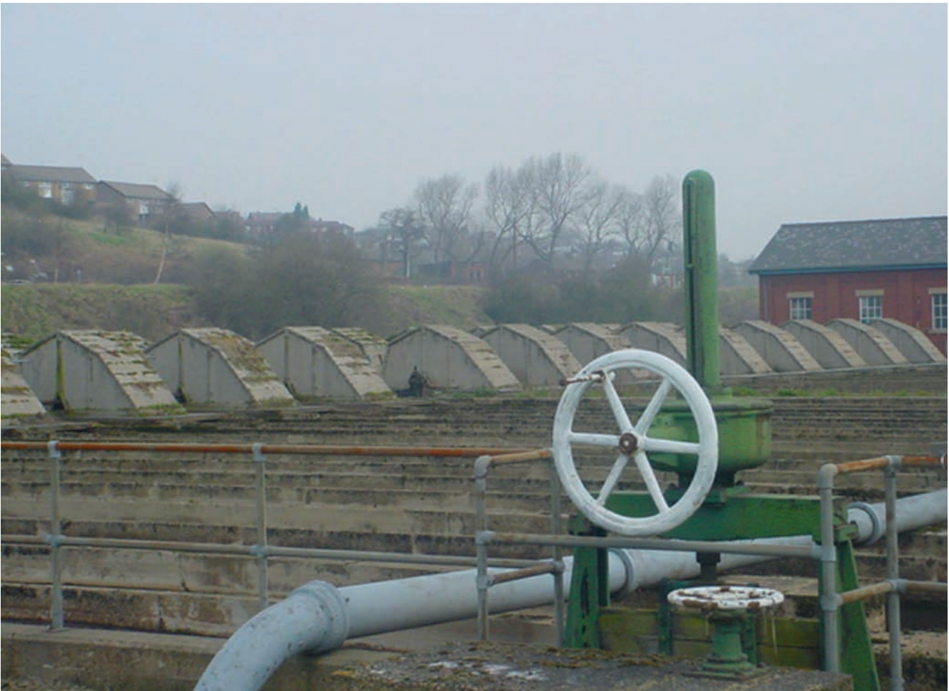
Calder Vale STW - Redundant Sheffield Units await demolition (April 2003) (courtesy: MWH & Yorkshire Water Services Ltd).
