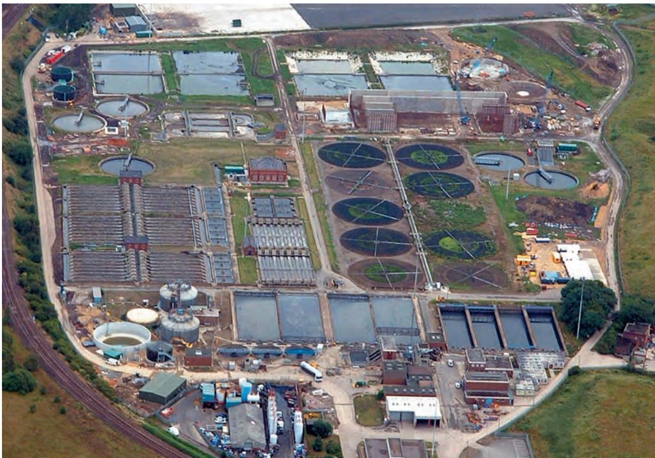
Calder Vale STW - aerial view of upgrades under construction (courtesy John Gruson BEng, BSc).
