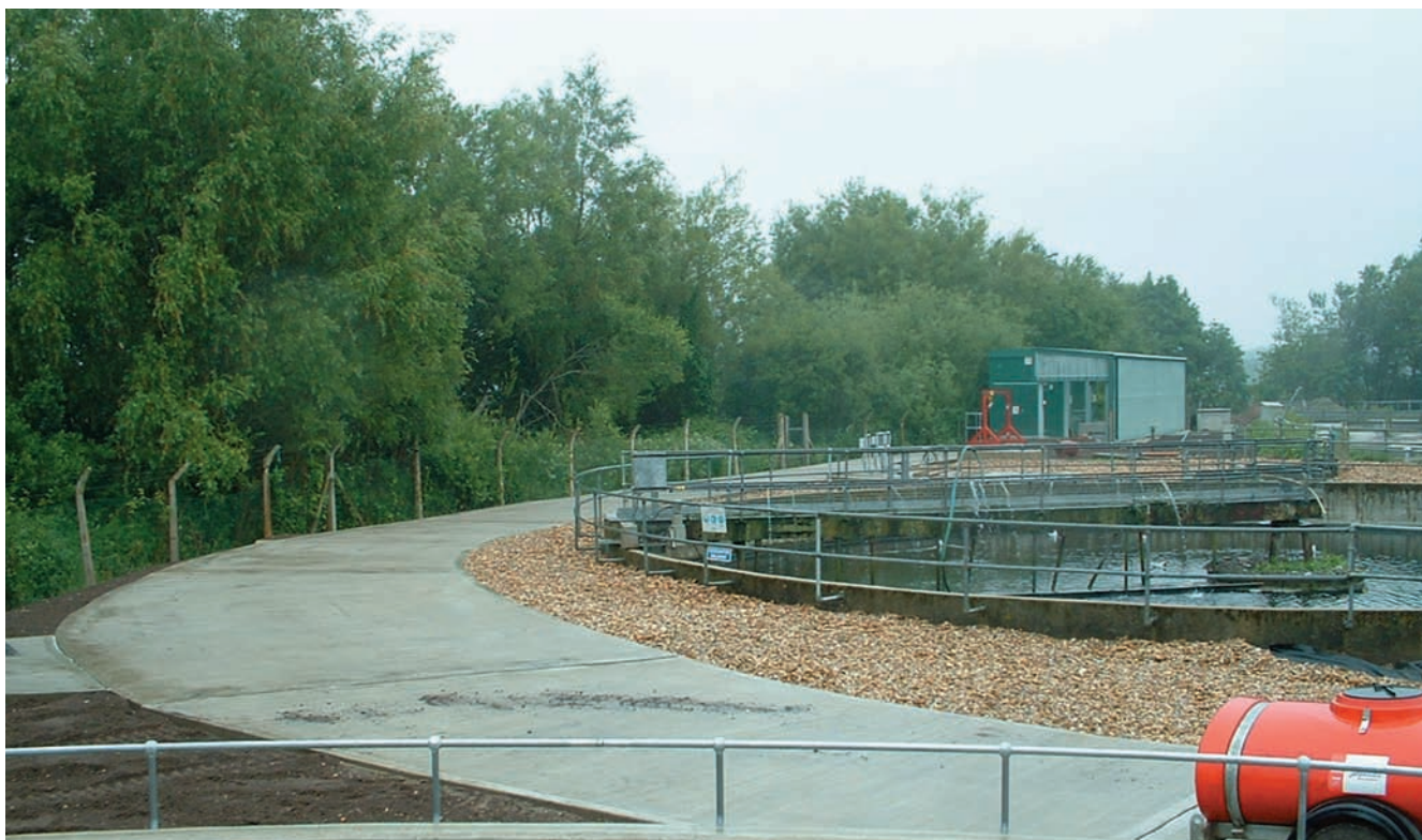
View of UV Installation (courtesy Wessex Water).
