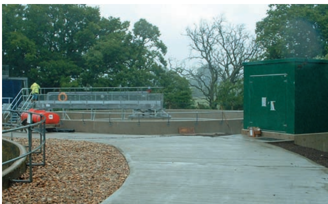
New storm tank (courtesy Wessex Water).
