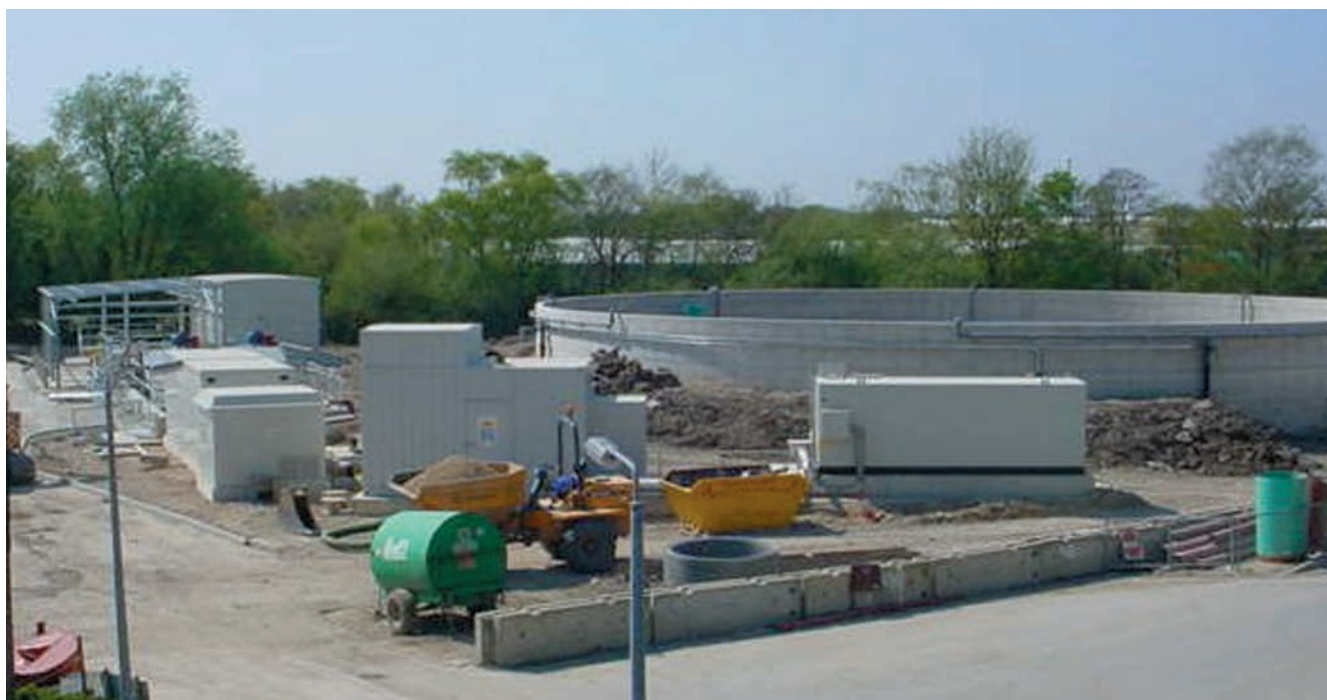
Poole WwTW storm tanks (Wessex Water Engineering Services).
