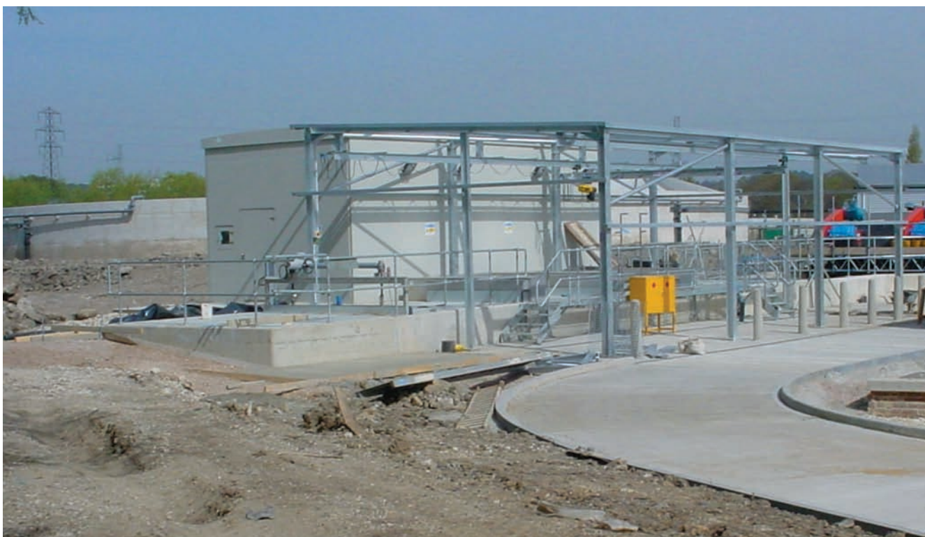
Poole WwTW UV plant (Wessex Water Engineering Services).
