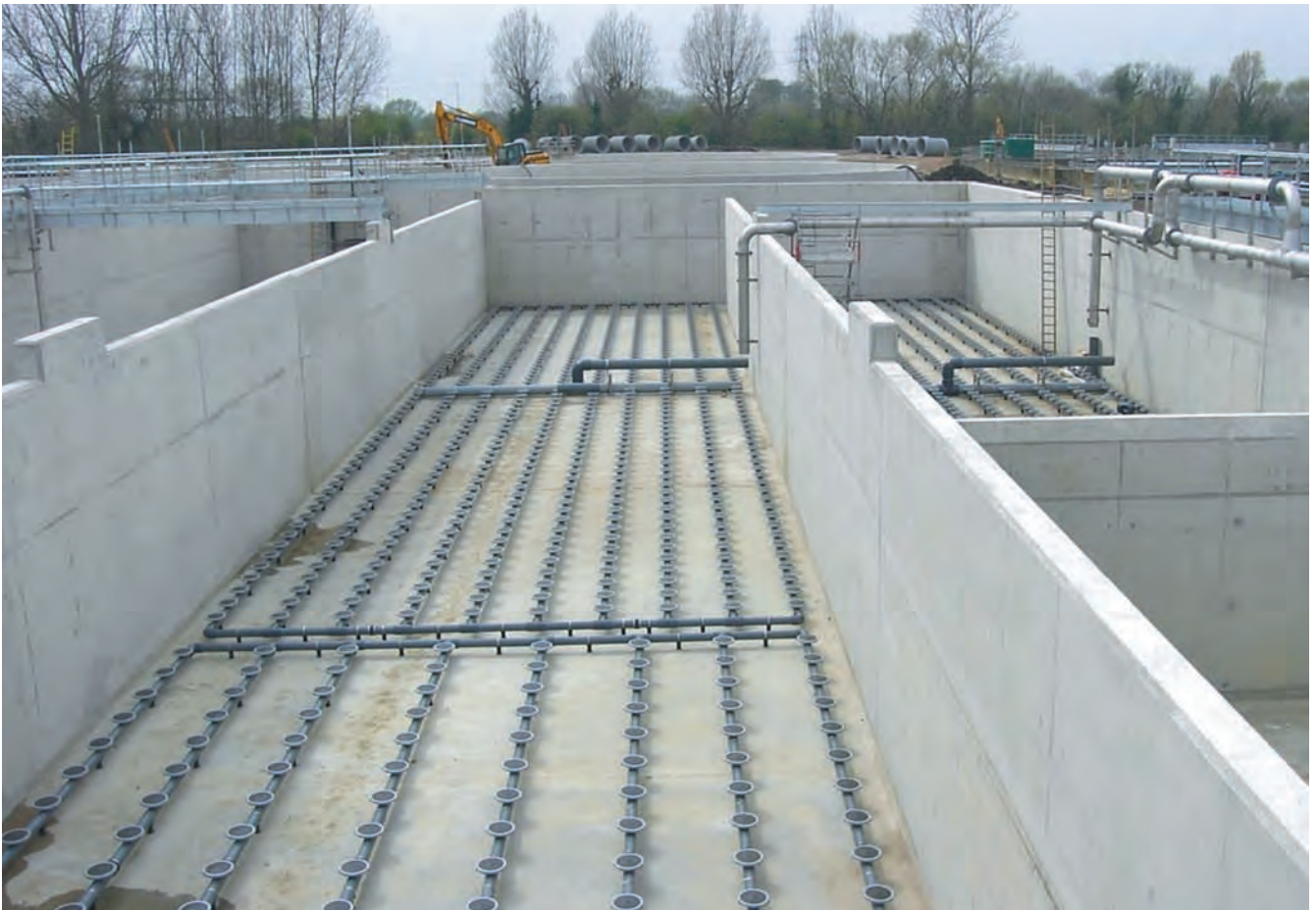
New aeration tanks with membrane diffusers (courtesy Thames Water Utilities Ltd)
