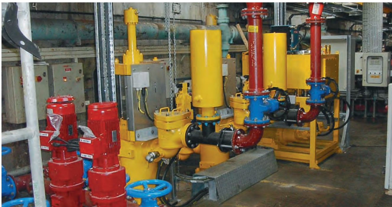
Refurbished primary de-sludging plant (courtesy Thames Water Utilities Ltd).
