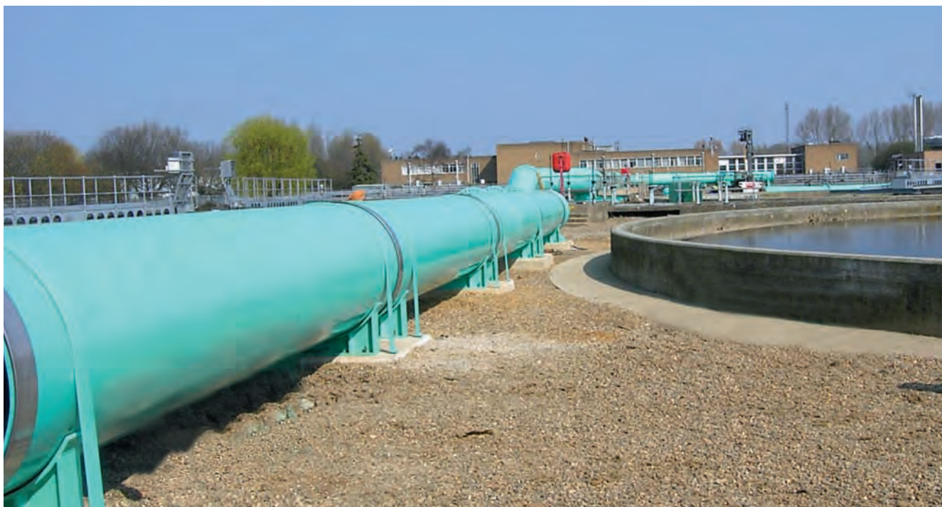
New air distribution mains to existing treatment diffusers (courtesy Thames Water Utilities Ltd).
