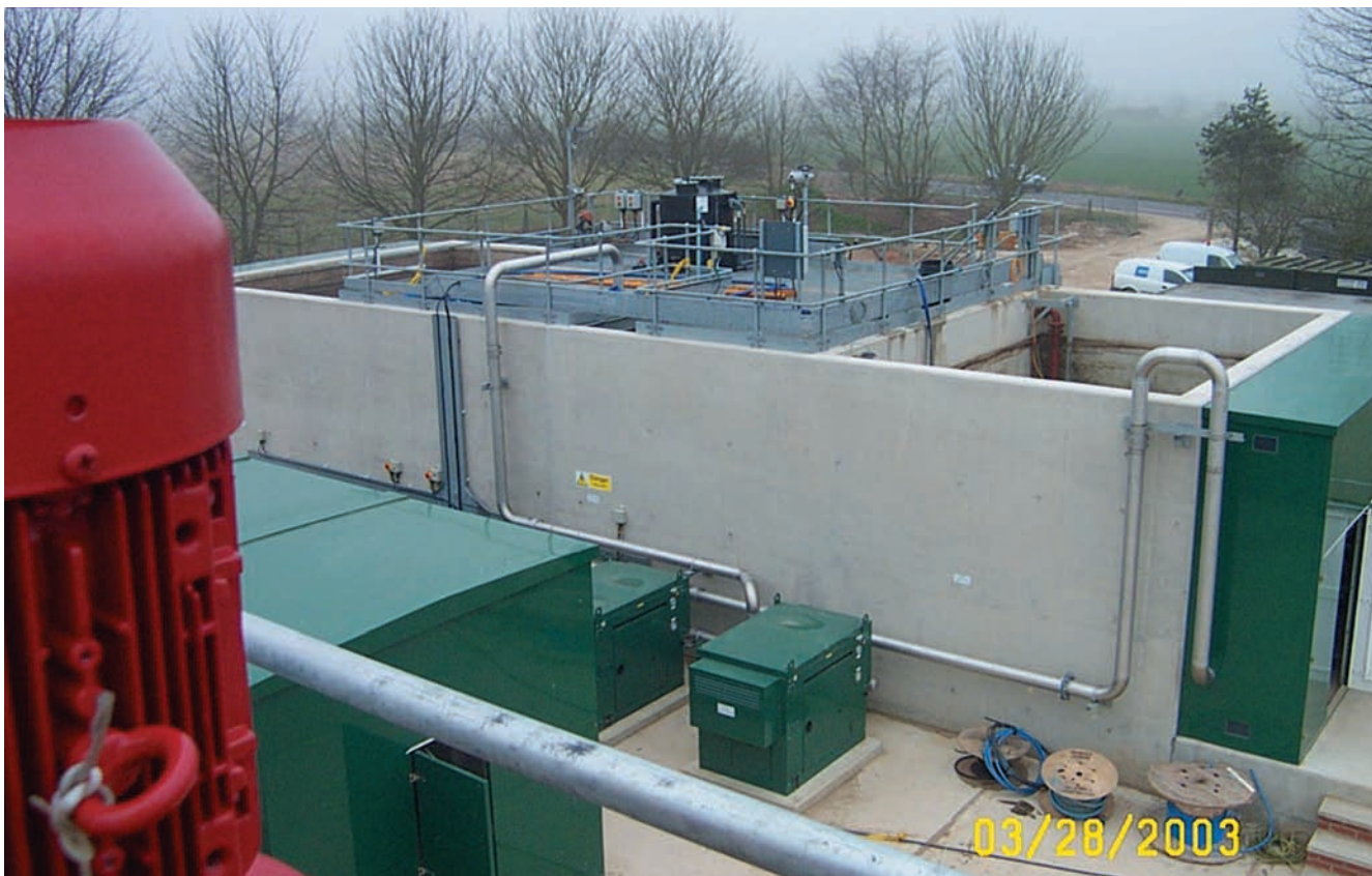
Skipsea WwTW MBR Plant (courtesy Eastern CaST)
