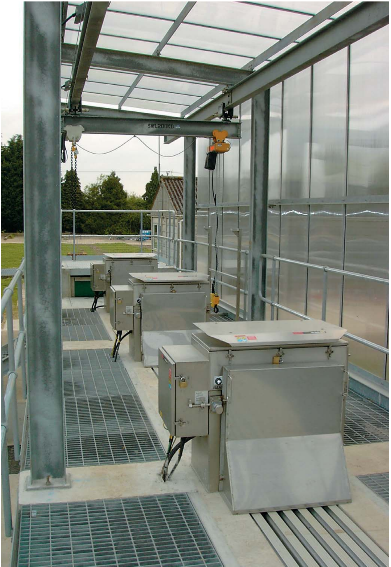
Tertiary UV disinfection at Wessex STWs
