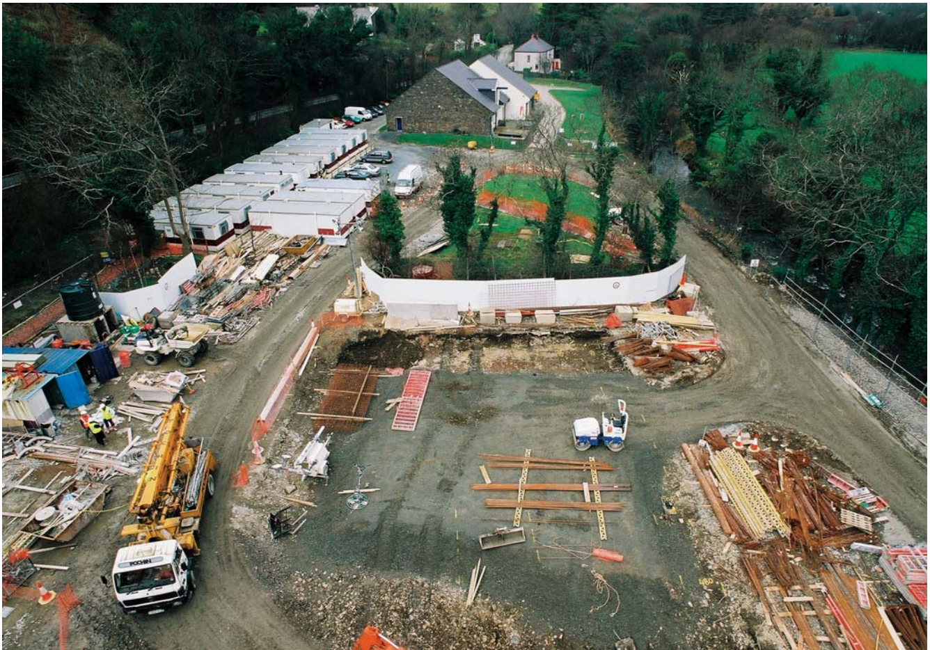
Sulby, IOM: Elevated view looking towards Gable end of existing works; chemical storage area prior to construction in foreground; river to right and retention of mature trees. photo courtesy Earth Tech Engineering.
