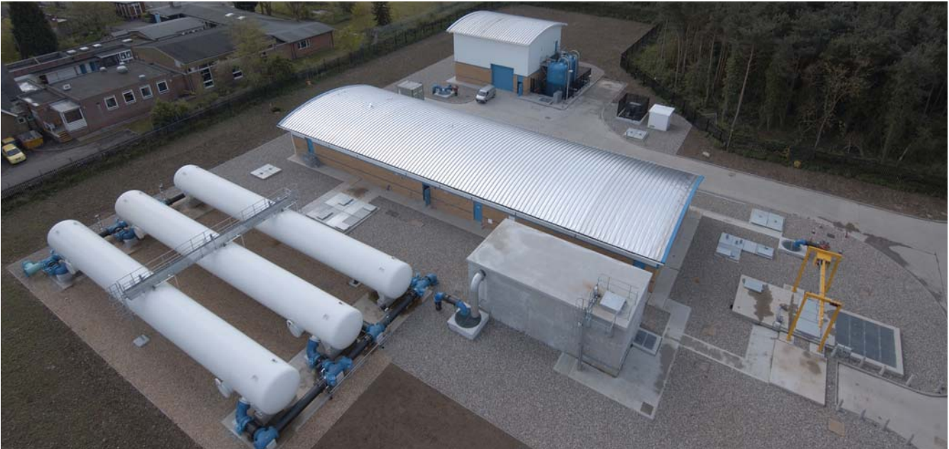
Aerial view of WTW site, Junior school at left and badger setts in woodland to rear
