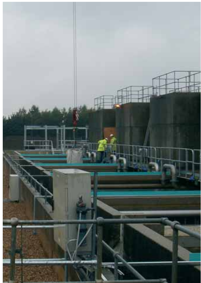
Media installation to Filter No.7 courtesy Essex & Suffolk Water & Mowlem PLC
