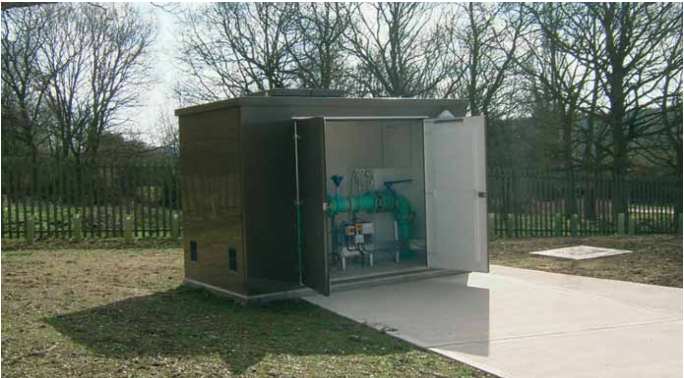
North Essex: Headworks of the New Borehole to supply 4.25Ml/d
