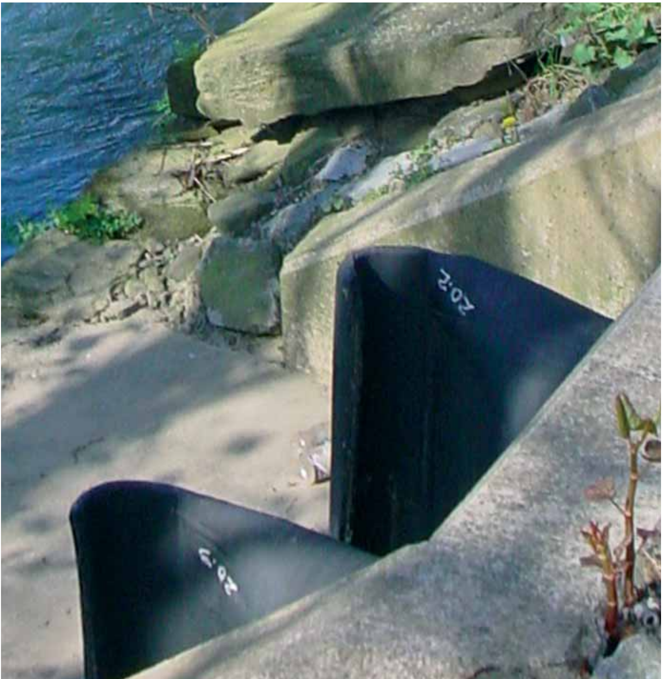
Rhymney: Outfall for improved CSO at Ystrad Mynach
