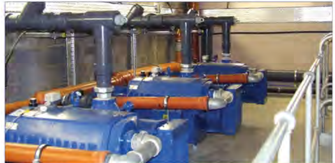
Located on Coast Drive in the Lade car park, this pumping station contains three 15kW pumps, a 20m 3 vacuum tank and a pneumatic discharge system.
