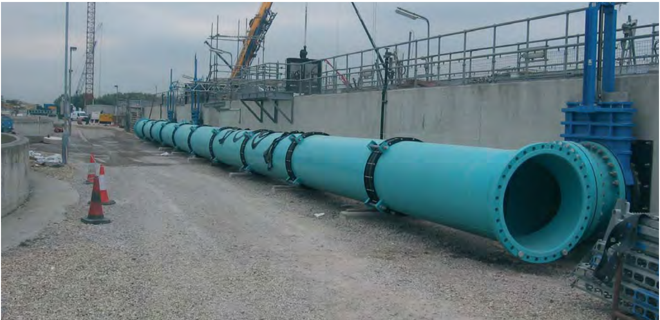
ASP No 1 & No 2 connecting pipe
