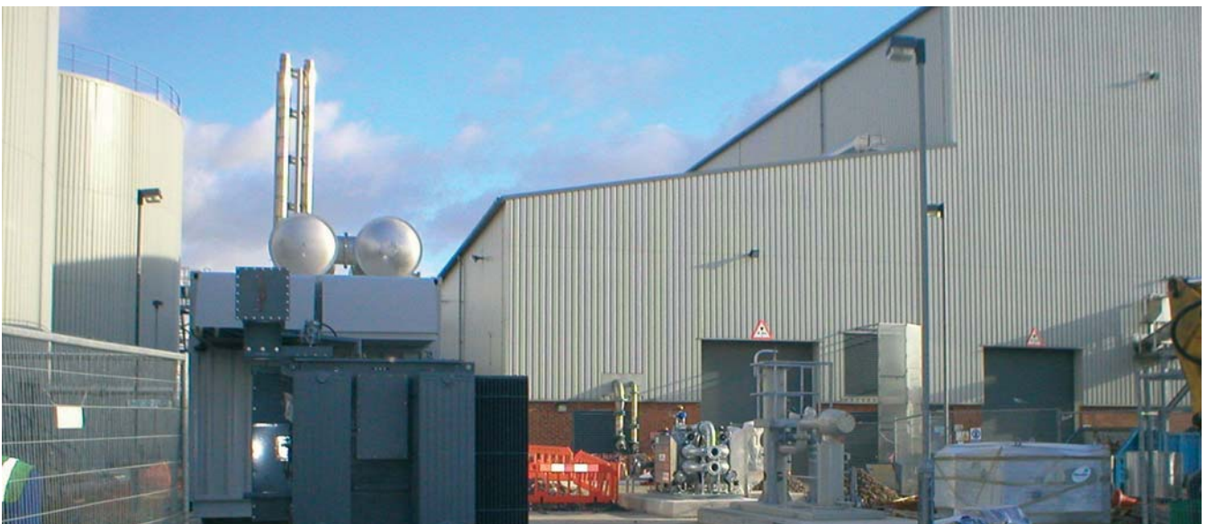
Carbon Policy manager Martin Ross at Southern Water's CHP facility
