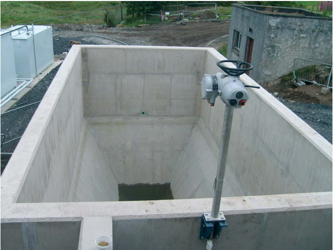
Coursehouse WTW - New Washwater Recovery Tank
