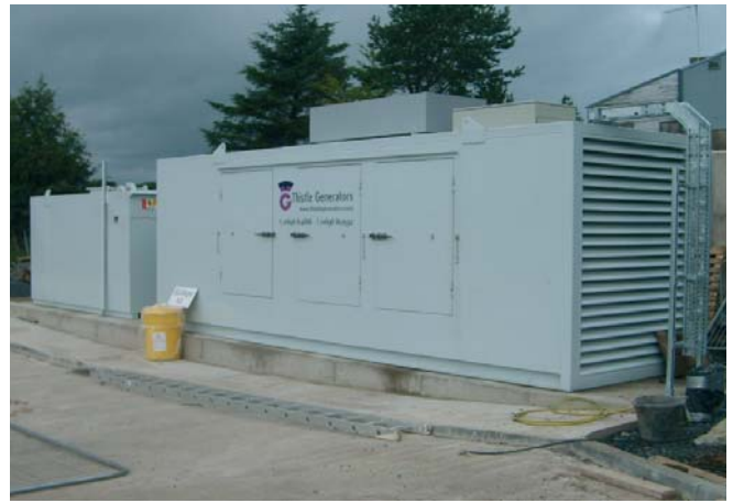
Coursehouse WTW - generator
