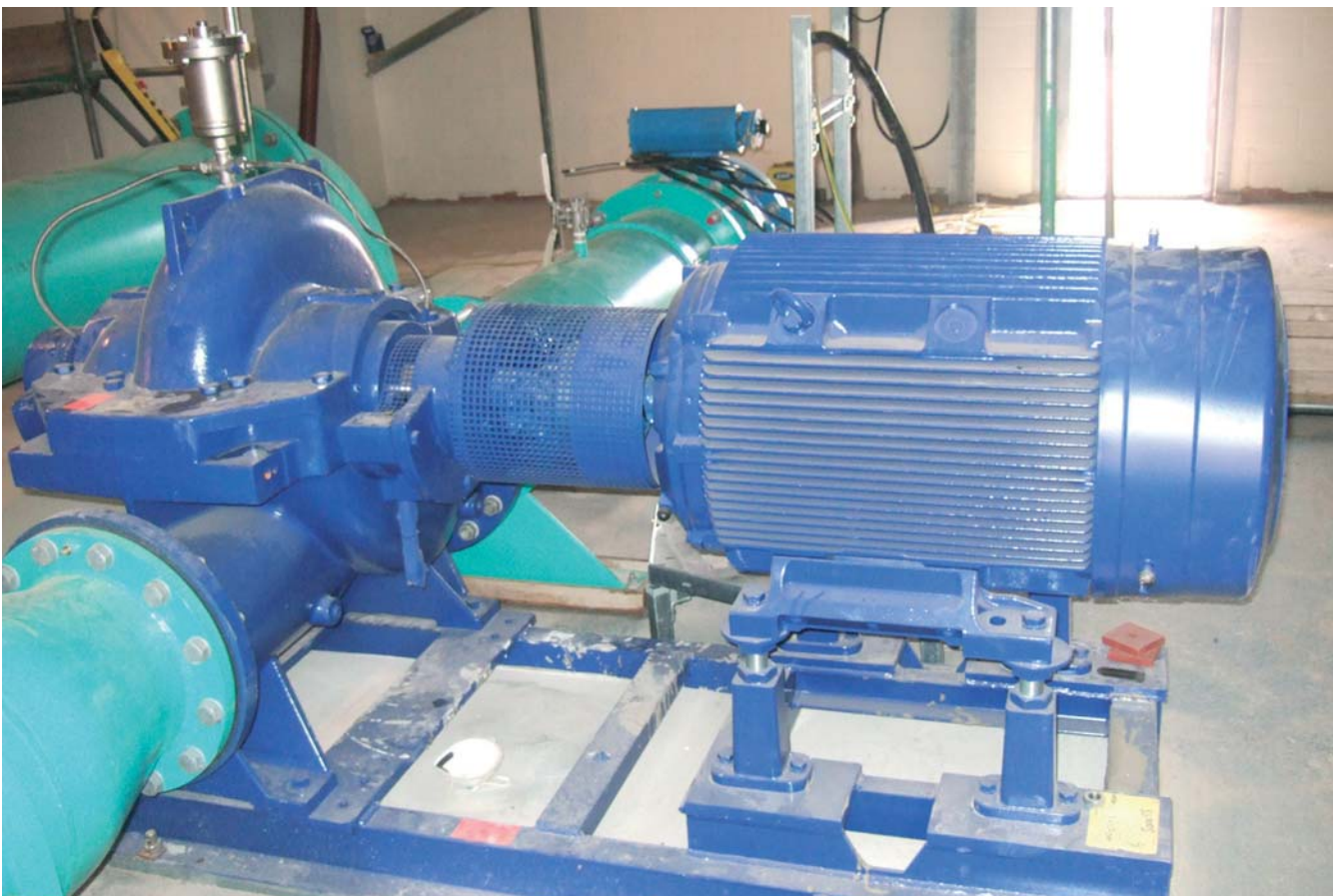
Steventon Pumping Station - Pump Set
