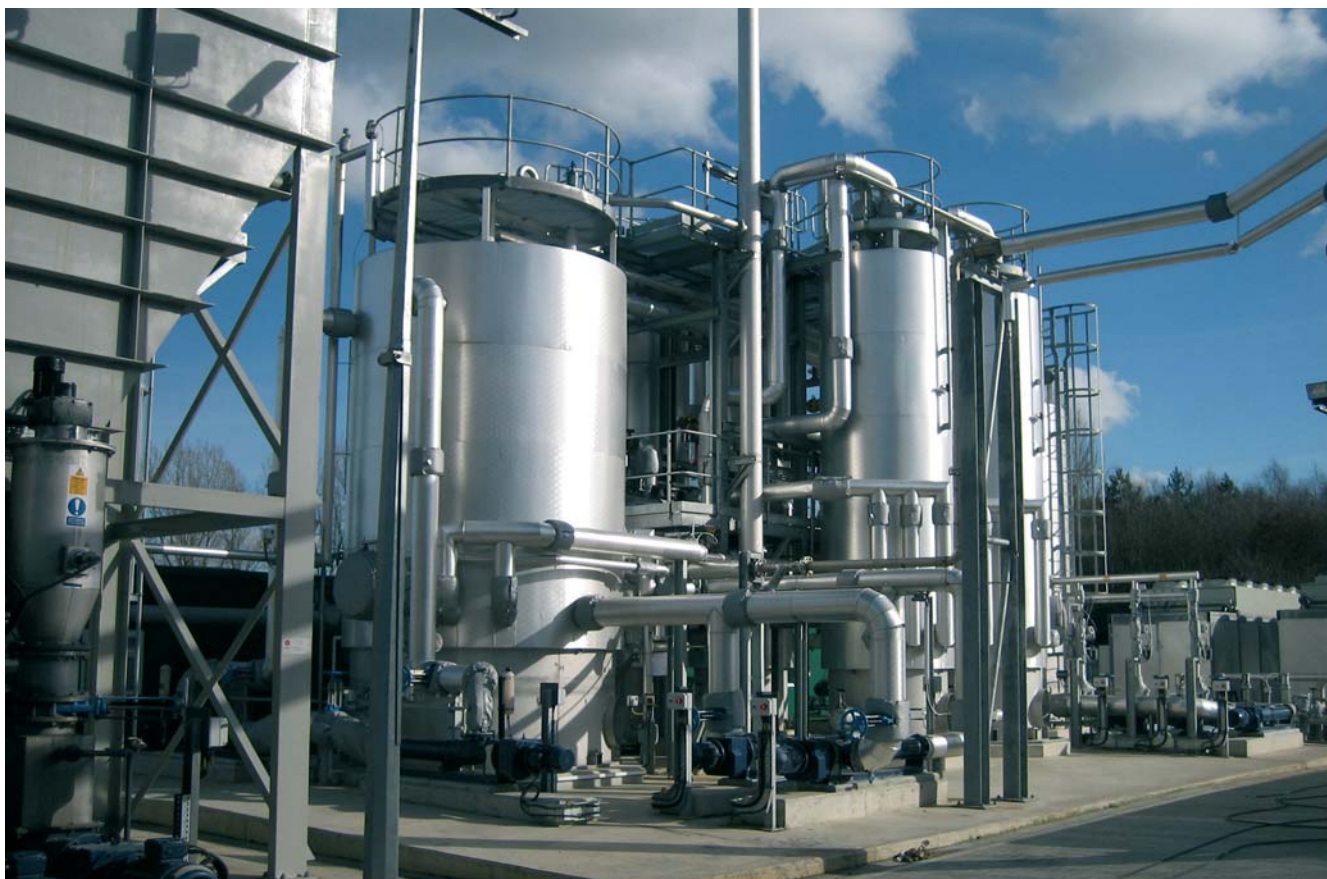
Cotton Valleys Cambi thermal hydrolysis plant with small footprint
