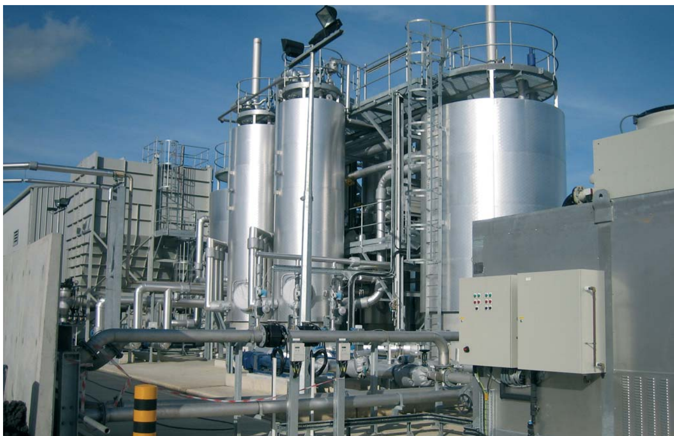
Cotton Valley's thermal hydrolysis plant - system demanded small space
