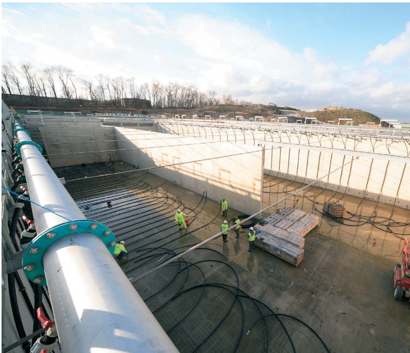
Installation of aeration pipe work in the new Activated Sludge Plant at Knostrop WwTW
