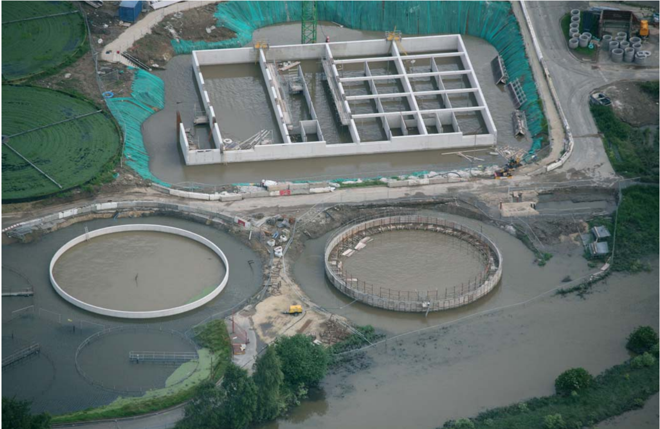
Aerial photo of new works at Lundwood WwTW inundated by floods in summer 2007
