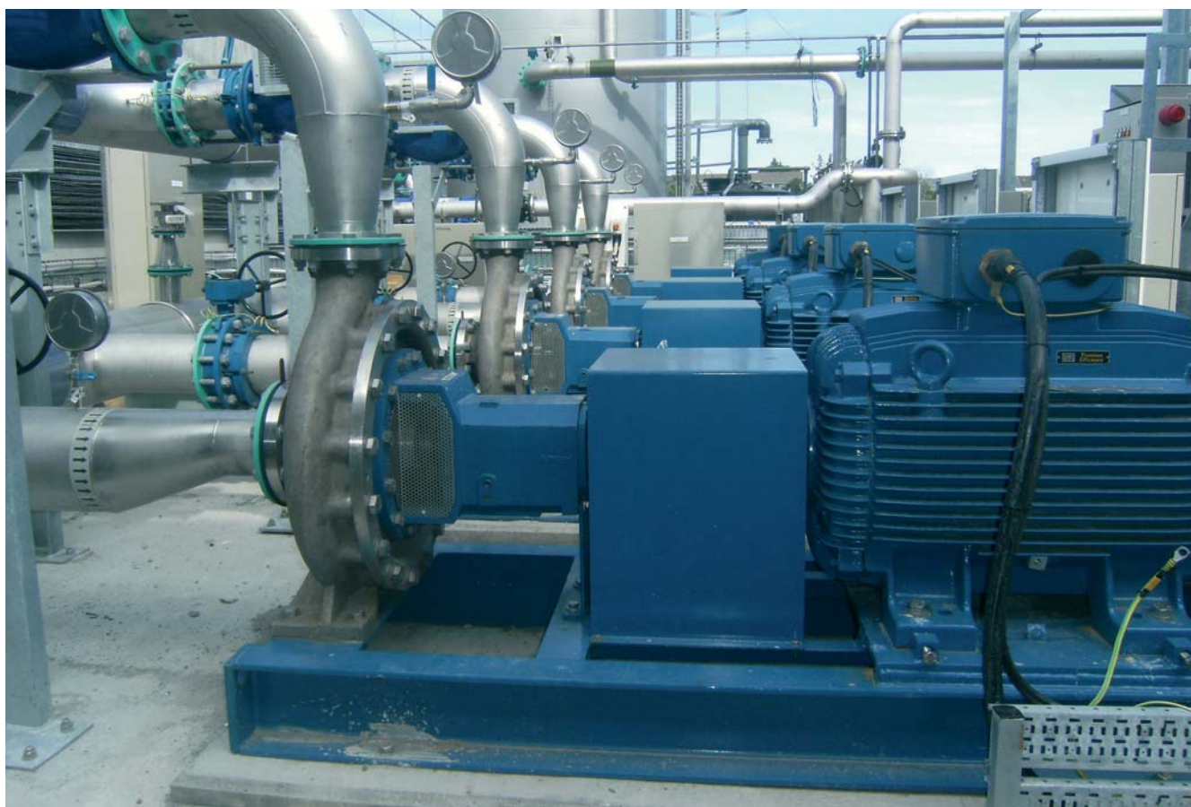
Longue Hougue treated water pumps with CIP tank in background
