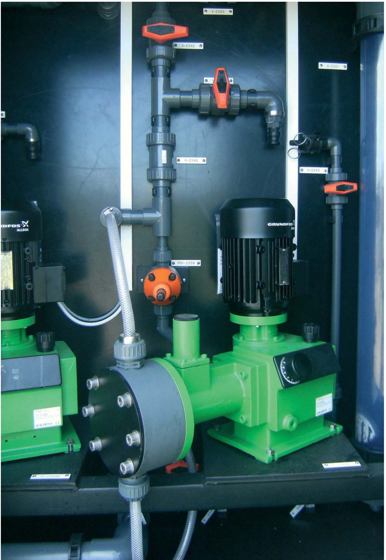
Longue Hougue Sodium Hypochlorite dosing pump
