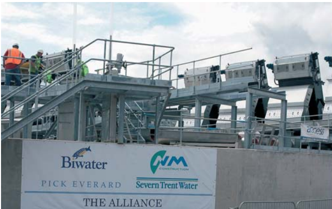
Photo shows the inlet works (left) & the 8 Fine Screens (right)
