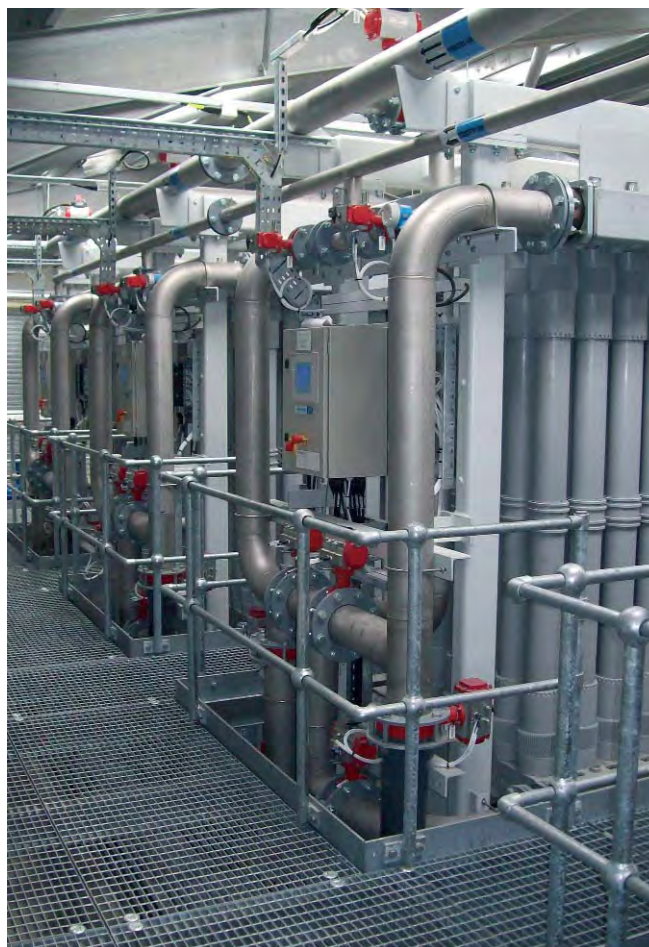
Membrane treatment plant - control panel view
