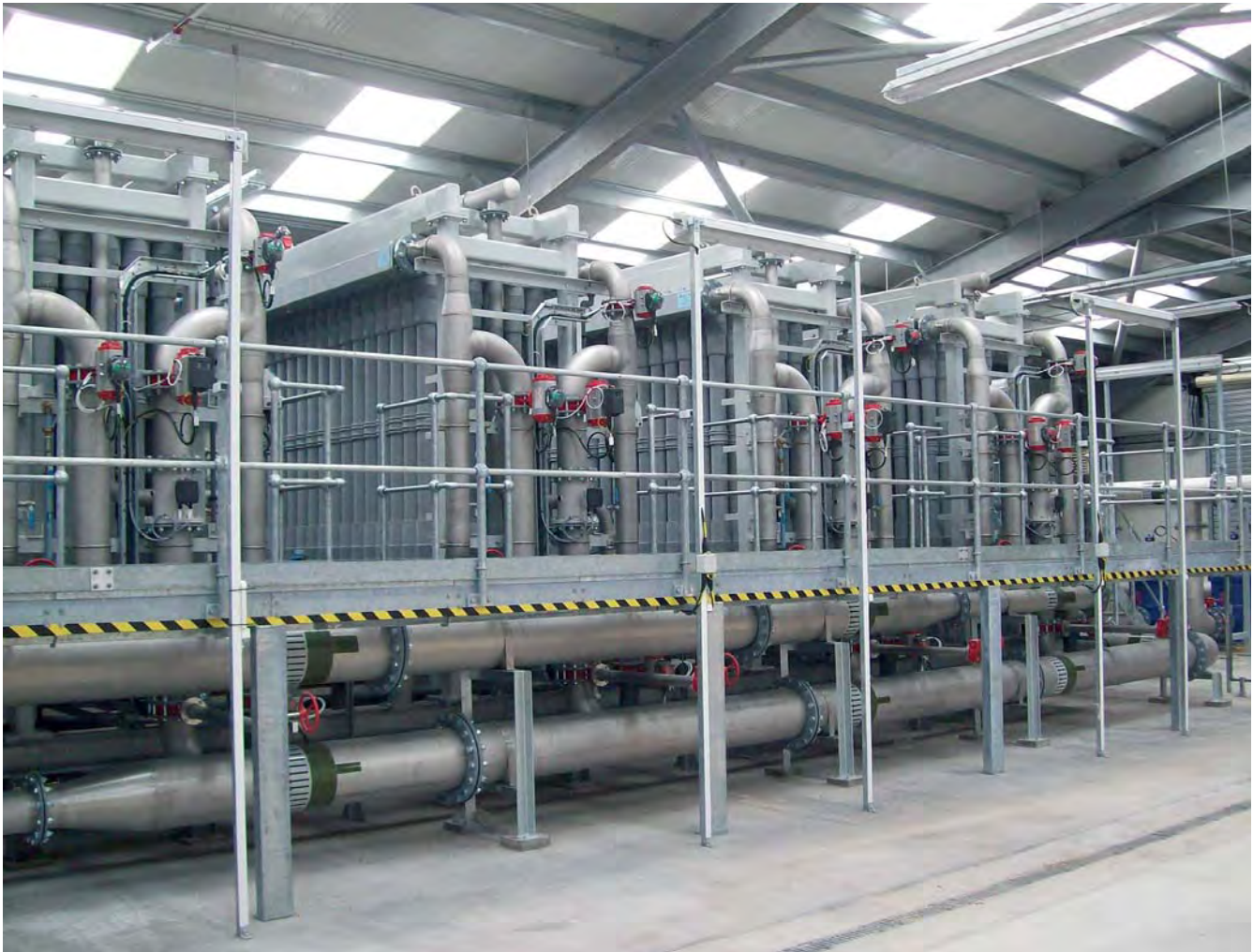
Membrane treatment plant - module assembly view
