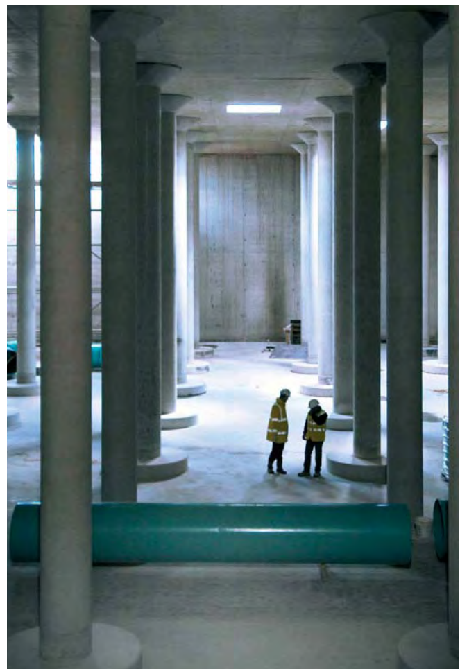
Inside one of the two new reservoir cells at Beacon Hill in Oxfordshire
