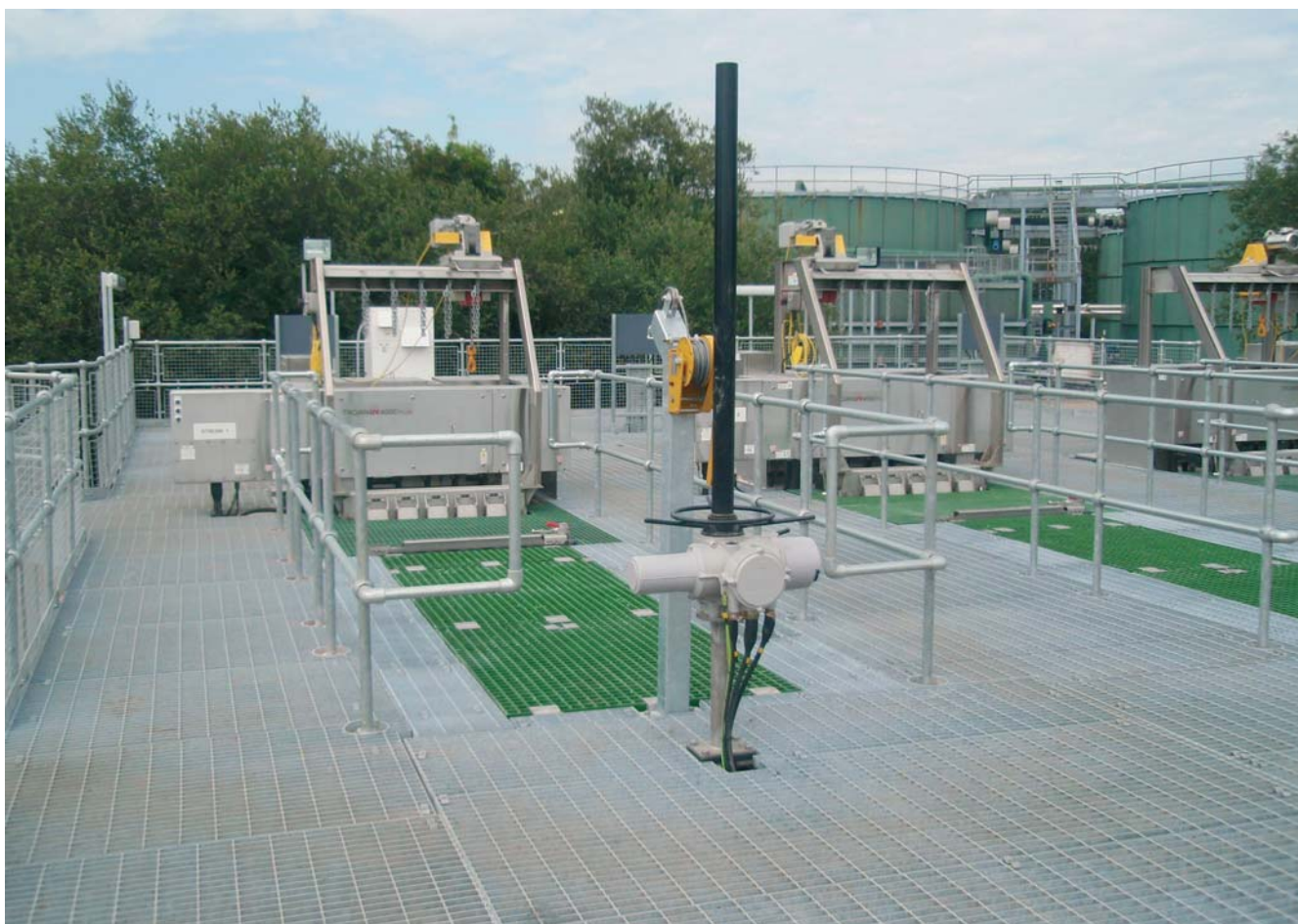
The 3 (no.) UV 4000 treatment banks installed
