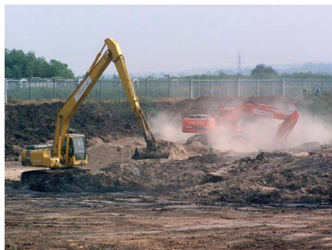
Emptying sludge lagoons. Sludge was mixed with saw dust and green waste prior to conditioning and ultimately use for landscaping applications around the region
