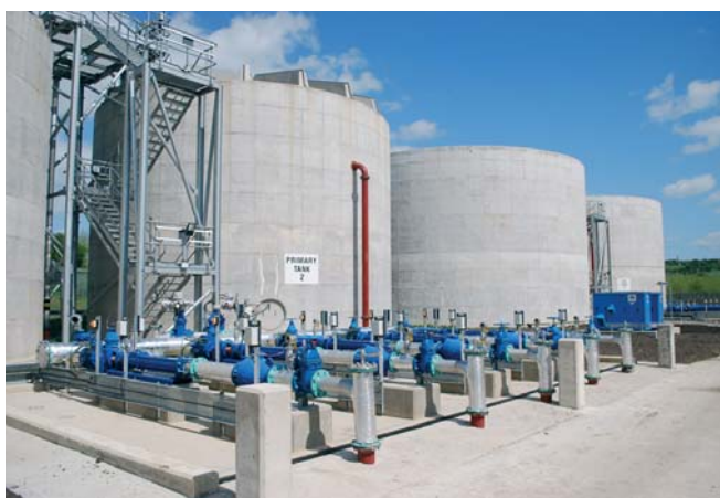
Mitchell Laithes – Sludge storage tanks and associated pumps and pipework
