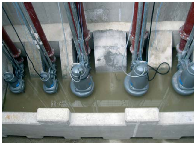
Harrogate WwTW - Internal view of the RAS/SAS pumping station
