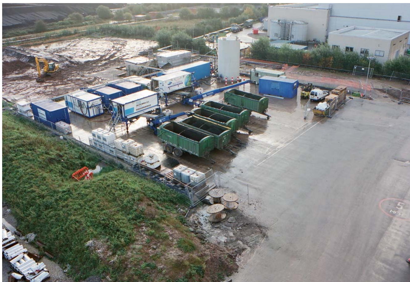
Mobile Temporary Dewatering Plant (Sept 2008)
