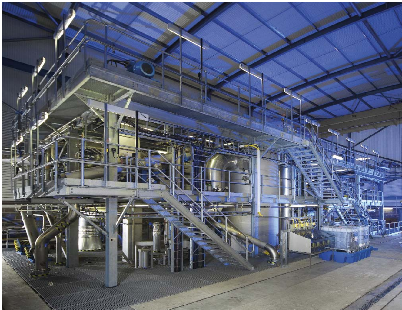
Ashford Sludge Treatment Centre
