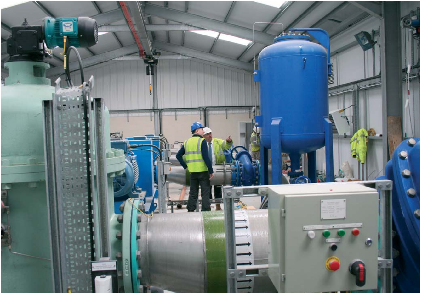
High lift pumping station
