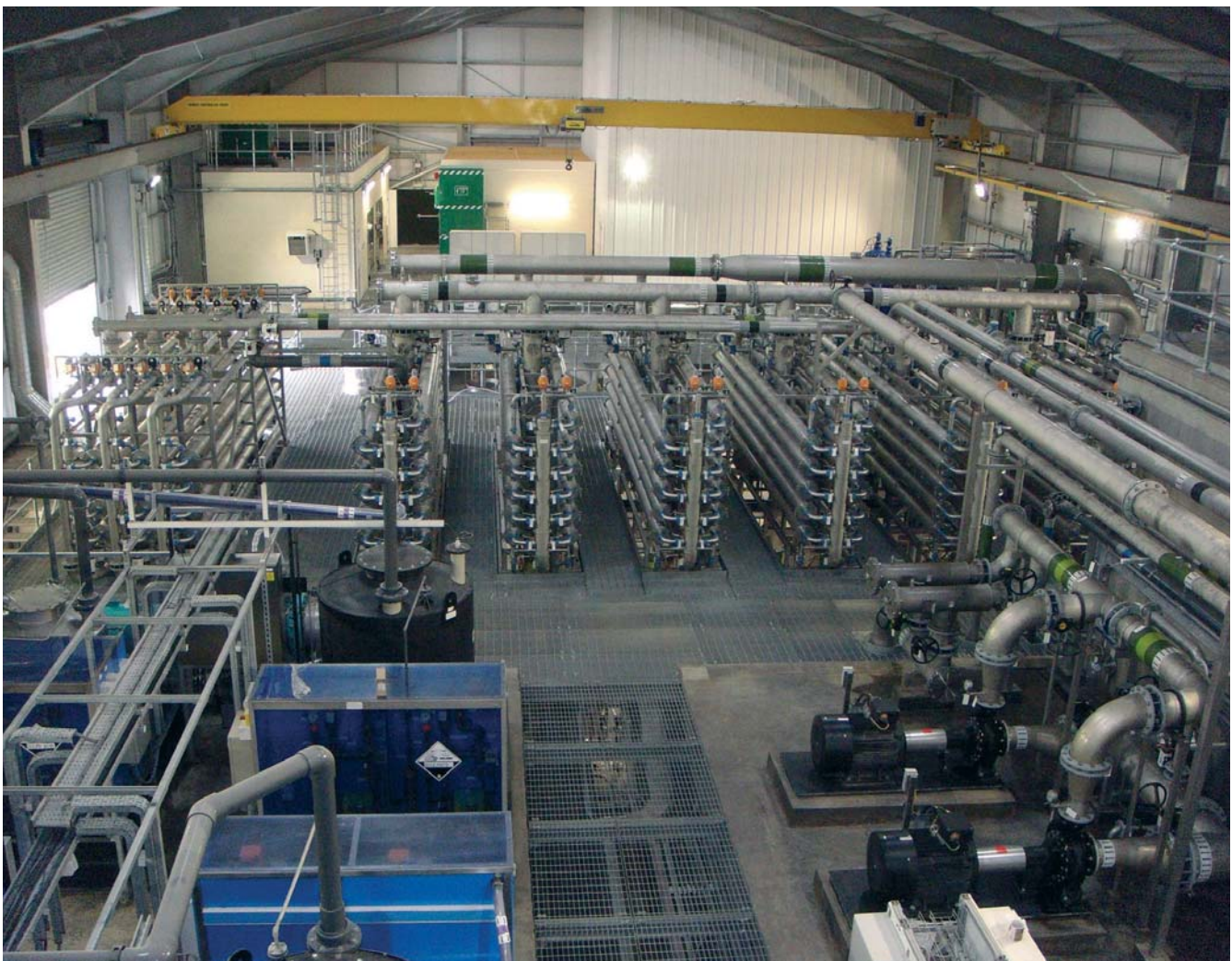
Membrane treatment plant
