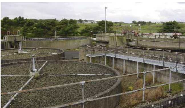
Some of the structures in the old Bushmills works which date back to the 1970s
