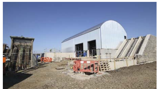
View showing the new screw pumps on right and old screws on left before they were demolished
