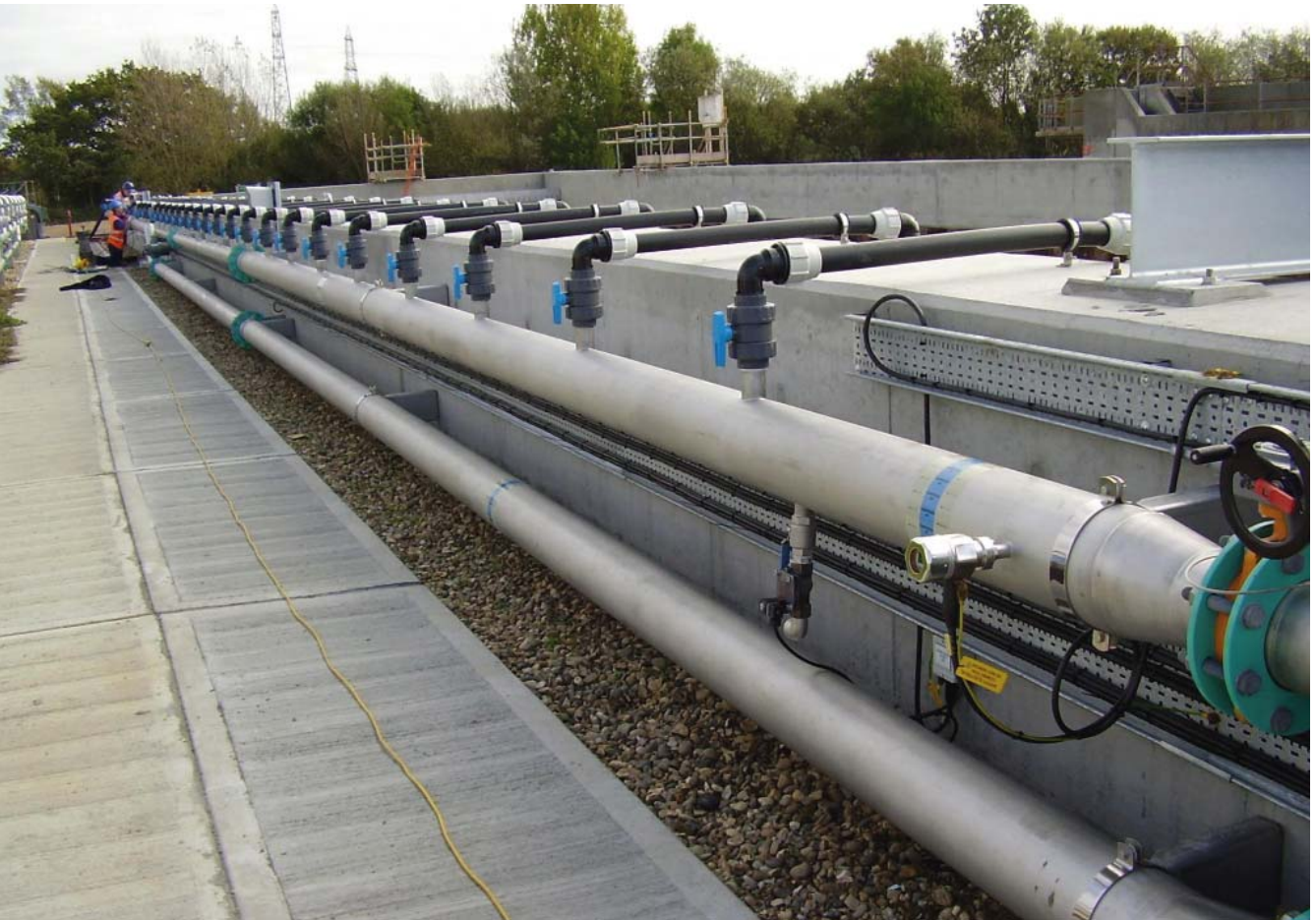
Aeration lane air pipework
