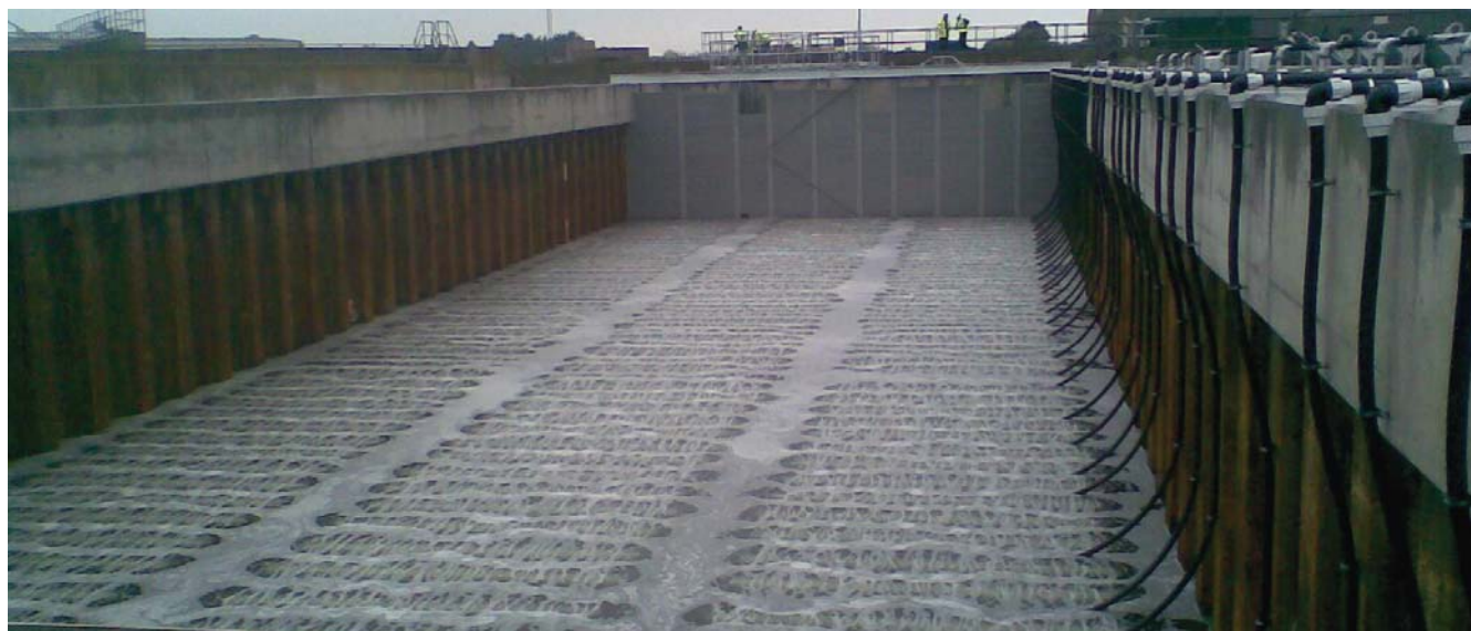
Aeration system pattern test
