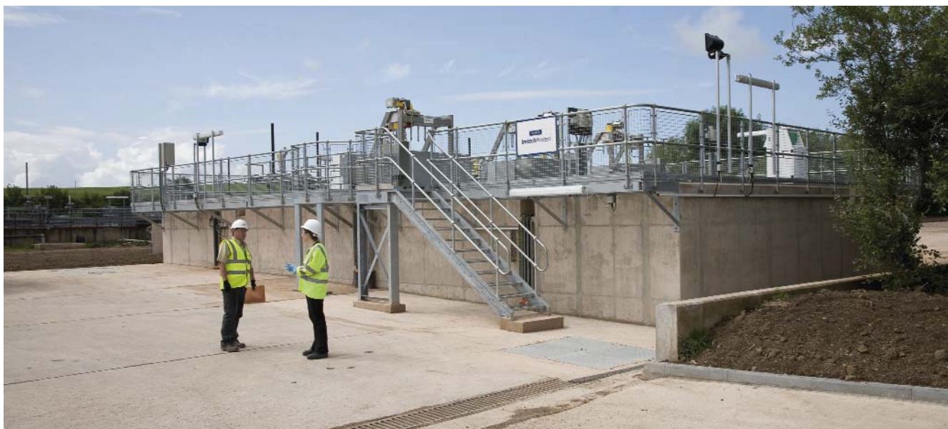
Cog Moors WwTW Storm UV Plant
