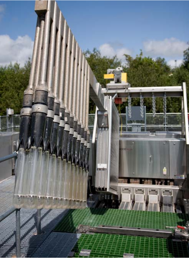
Single bank of 22 lamps, fitted with hydraulic wipers and static mixers. Lamps can be easily lifted for maintenance
