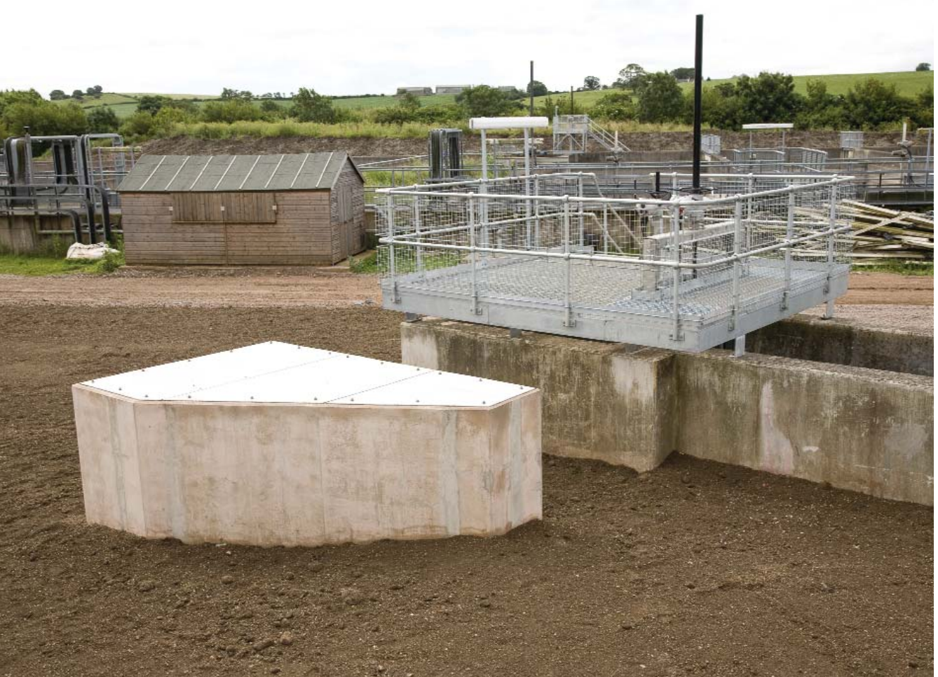
UV plant Inlet. The shed, rear left, housed the original pilot plant
