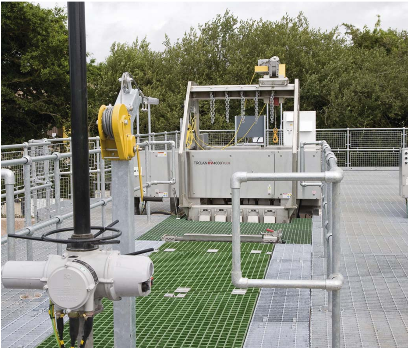
Trojan UV4000PLUS unit in situ. Channel lies below deck, inlet penstock control at front of photo
