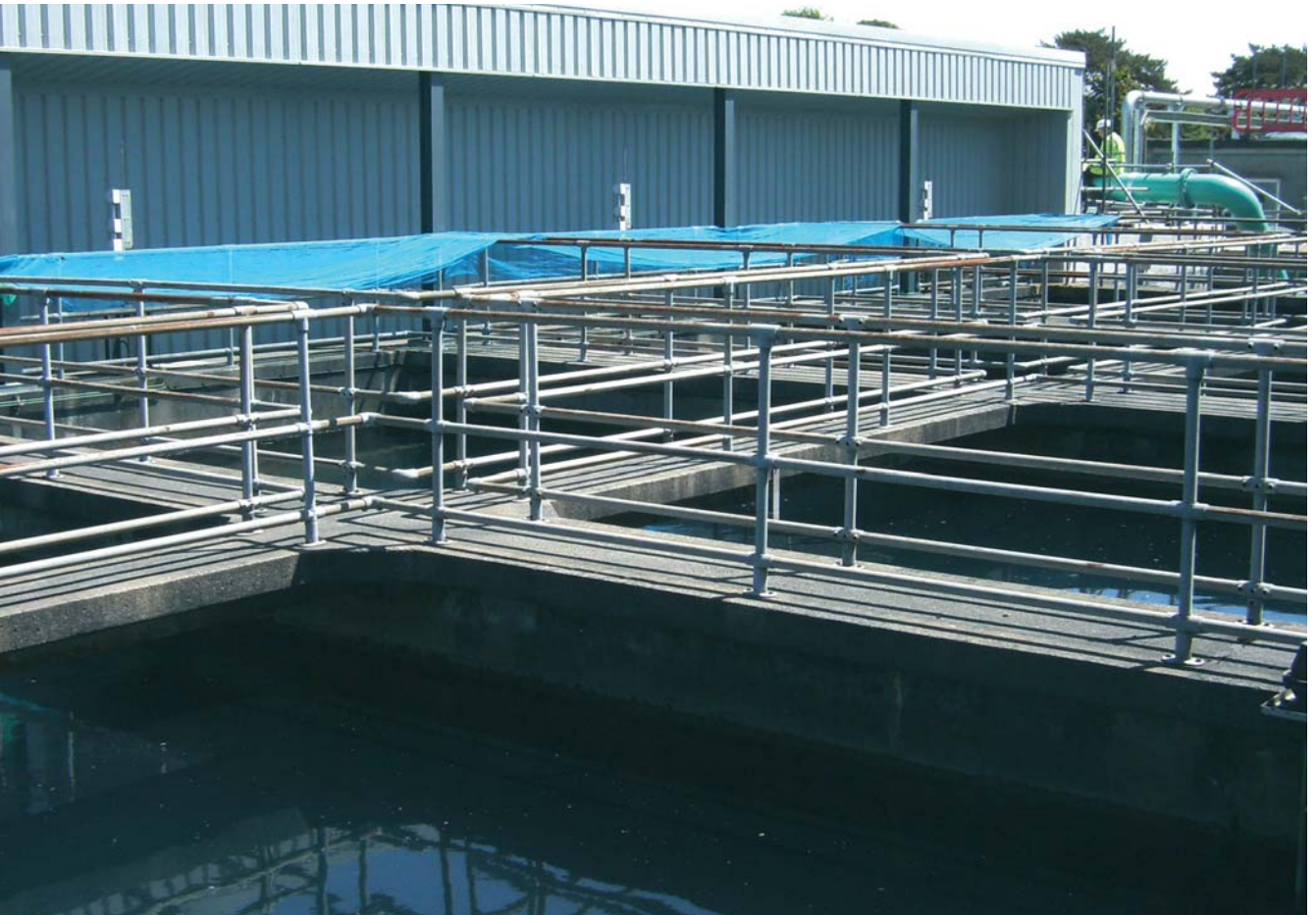
New backwash tank
