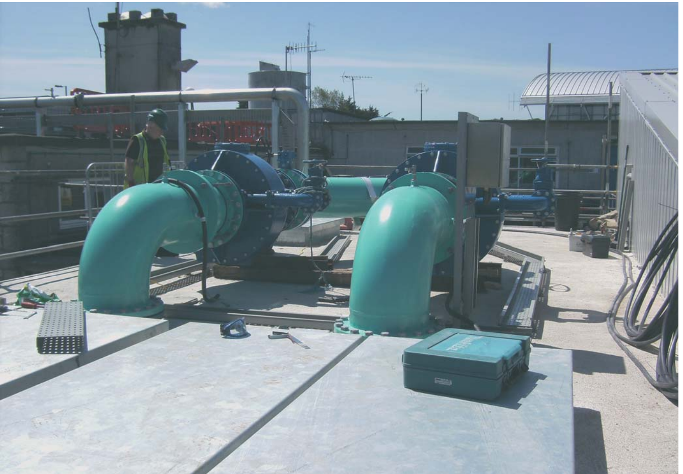
Backwash Pump Tank Discharge
